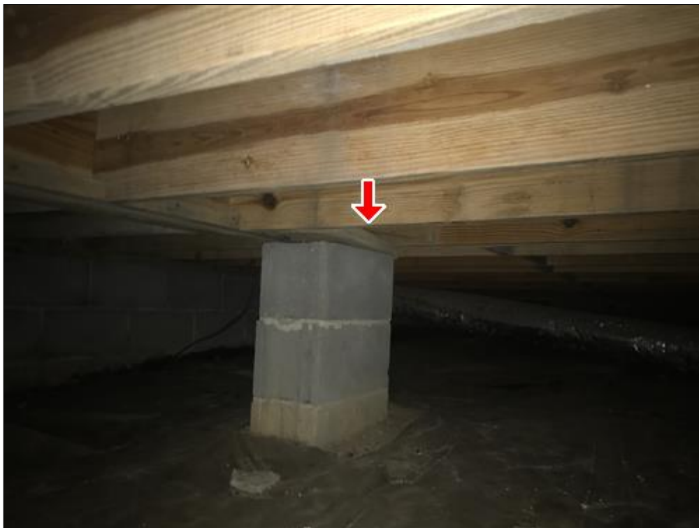
5.0 Picture 3 Wood cap loose
