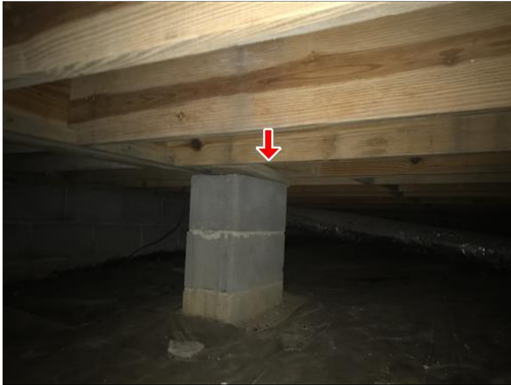
5.0 Picture 3 Wood cap loose
