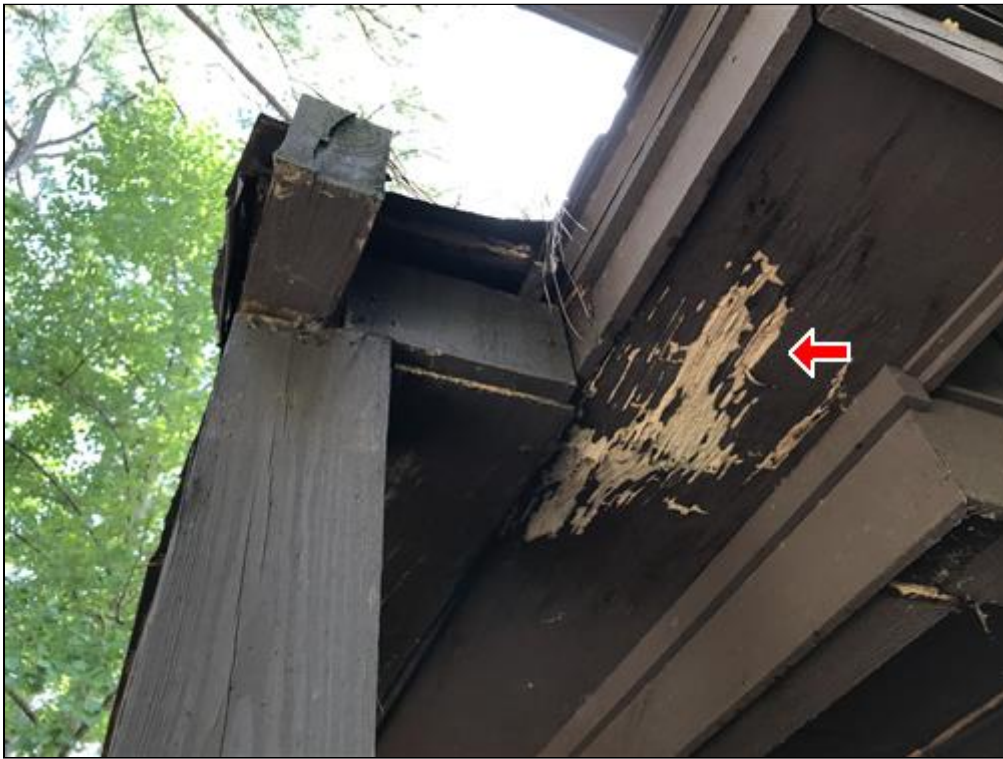
2.5 Picture 1 (possible termites)
