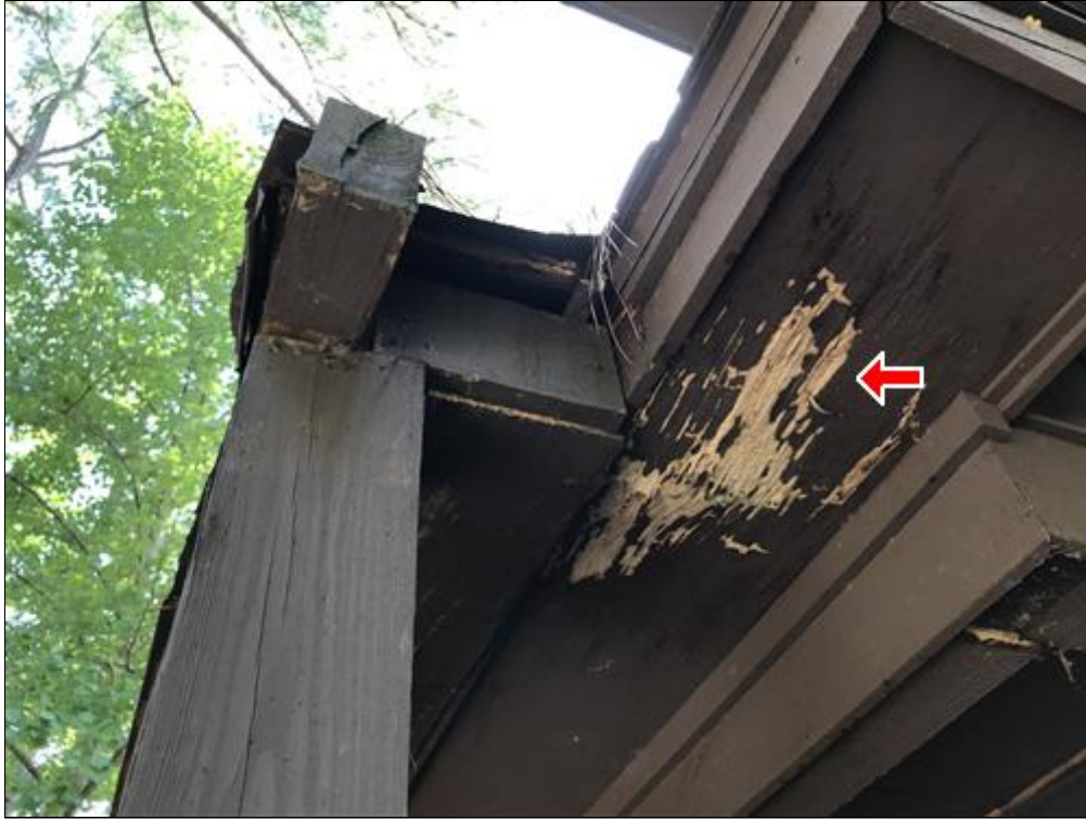
2.5 Picture 1 (possible termites)
