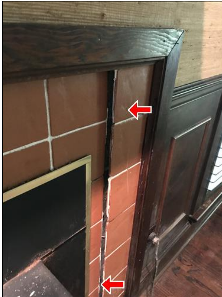
5.1 Picture 4 Signs that the fireplace is separating from the home.
