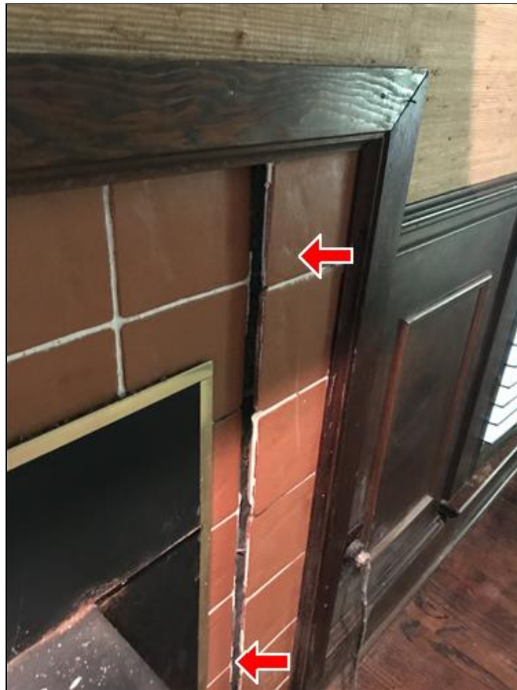
5.1 Picture 4 Signs that the fireplace is seperating from the home.
