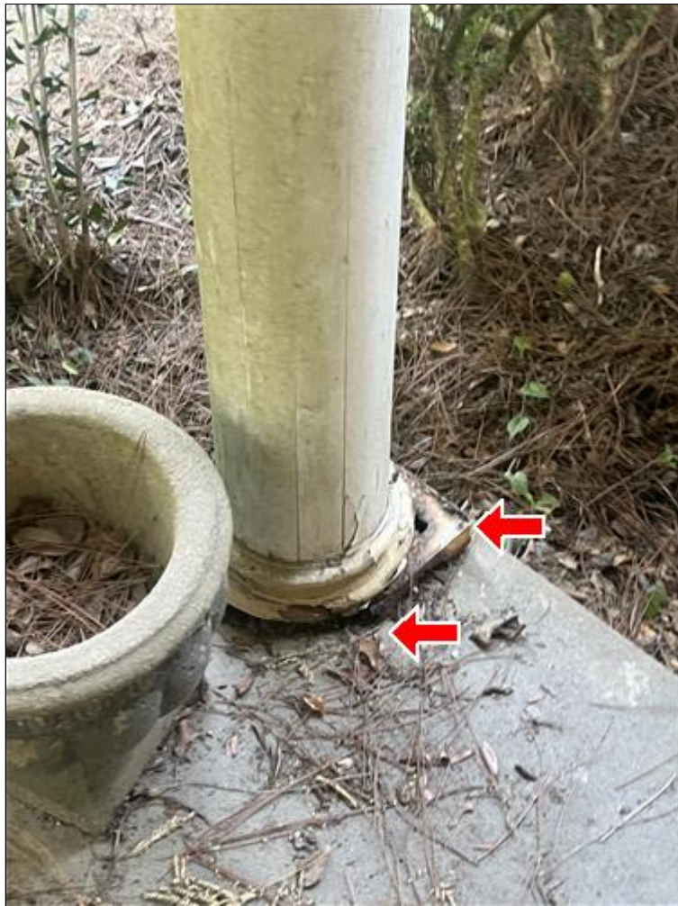
2.3 Picture 2 Trim deteriorated at bottom of column at front porch
