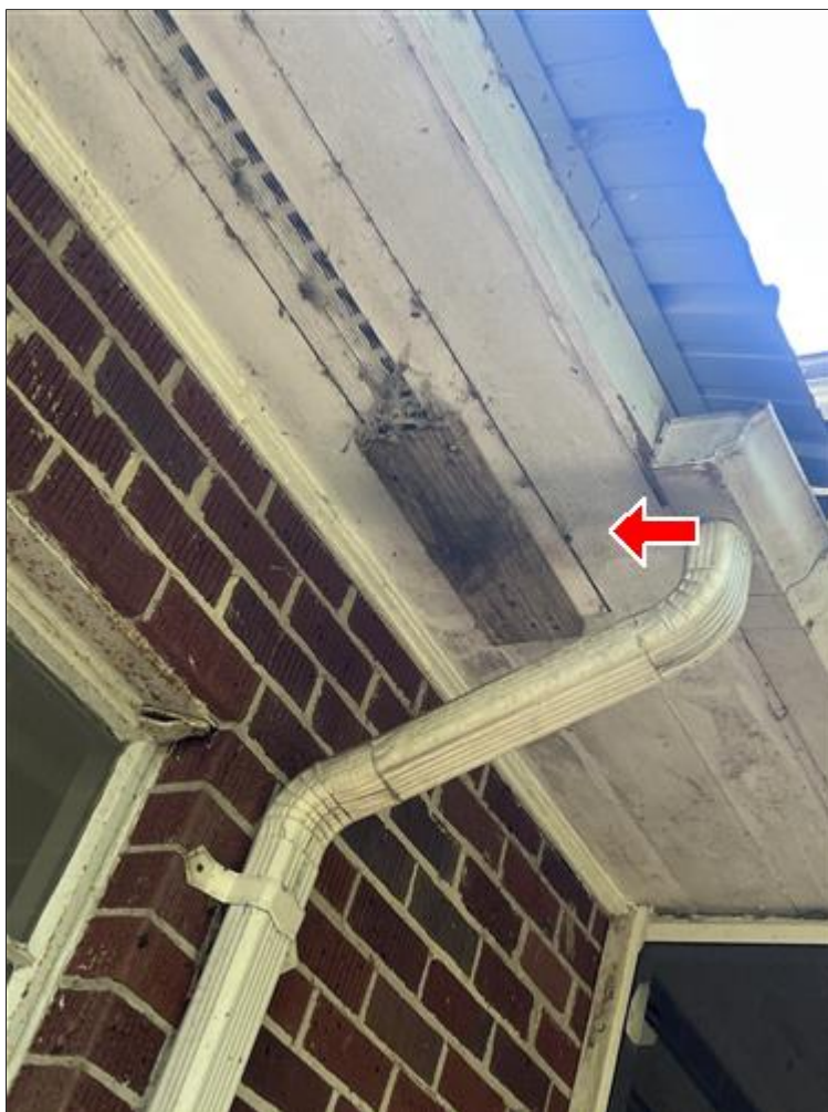
2.5 Picture 2 Repairs have been attempted at the rear of the home. This is just a patch not repaired correctly. This is for your information.
