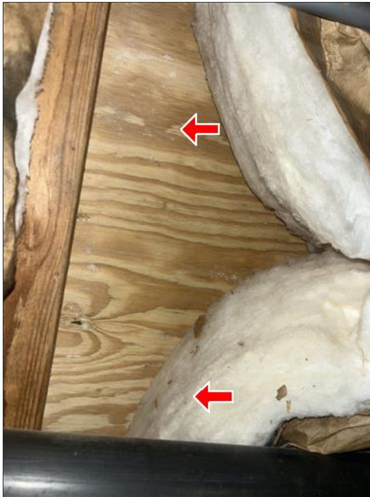
5.3 Picture 3 Past repairs made to the sub-flooring
