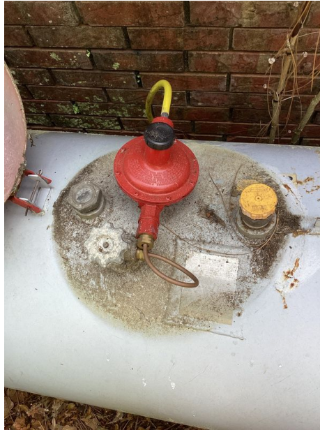
At LP Tank
