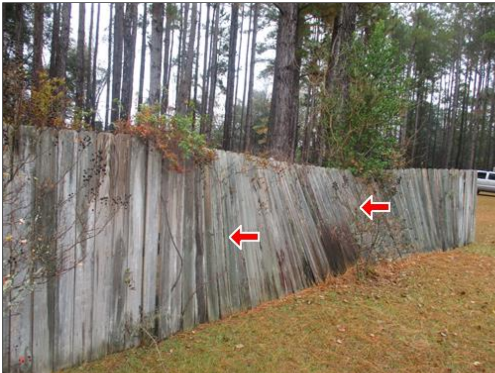
2.3 Picture 2 The wood fence is failing. A more proper support is needed.
