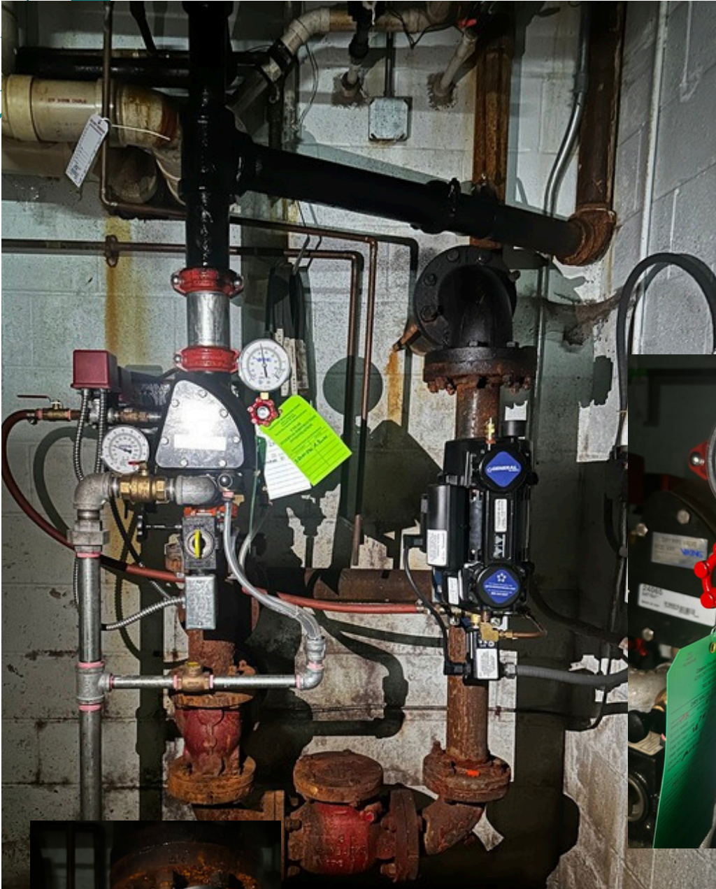
Industrial Dry Pipe Valve sprinkler system with inspection tags.
