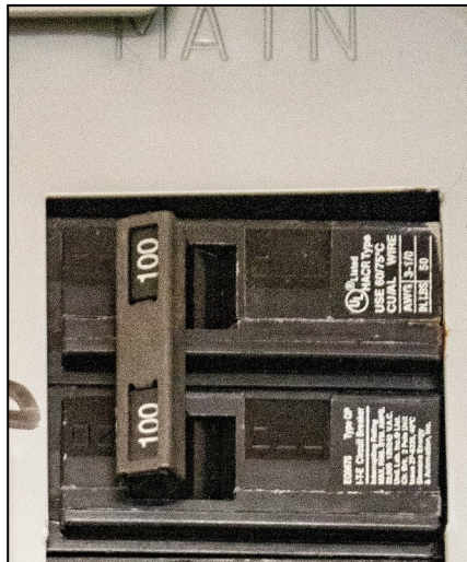
Electrical breaker box is located in the basement.
