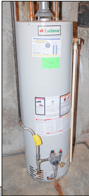
40 gallon, gas Lochinvar water heater with an inspection sticker dated 11-2-11.
