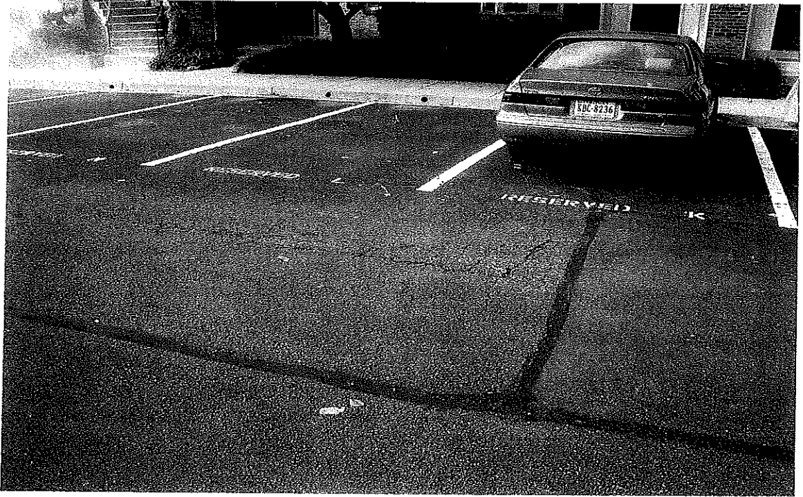
Previously filled asphalt cracks with new adjacent cracks.
