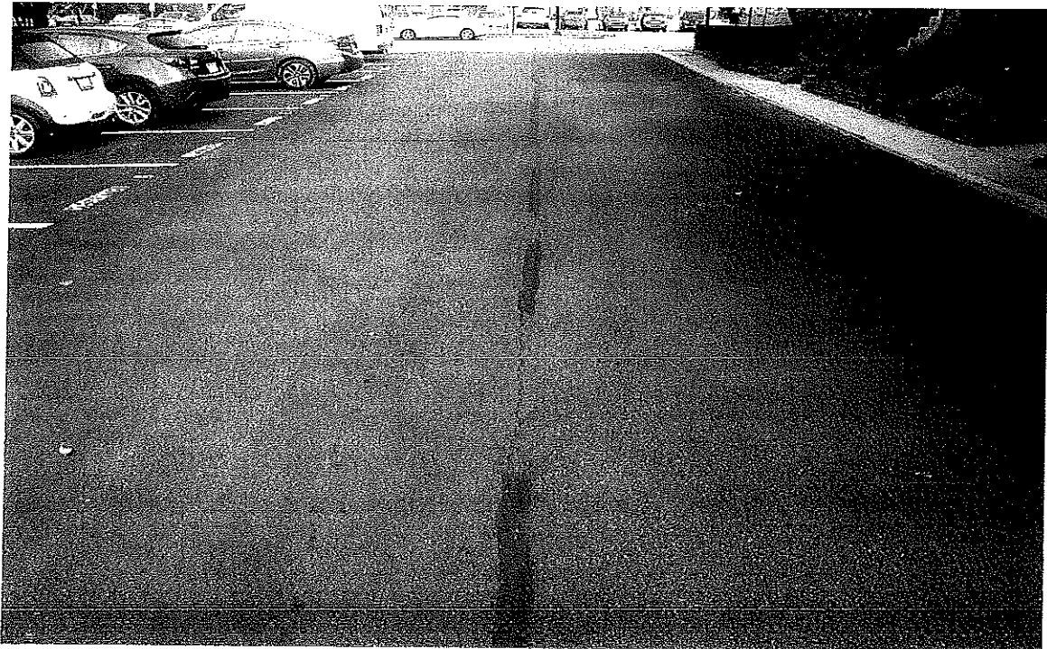
Another previously filled crack that has extended.
