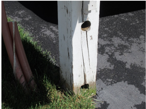
Paint finish and wood deterioration
