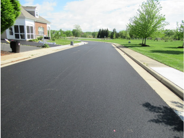
Fox Mill Way pavement overview
