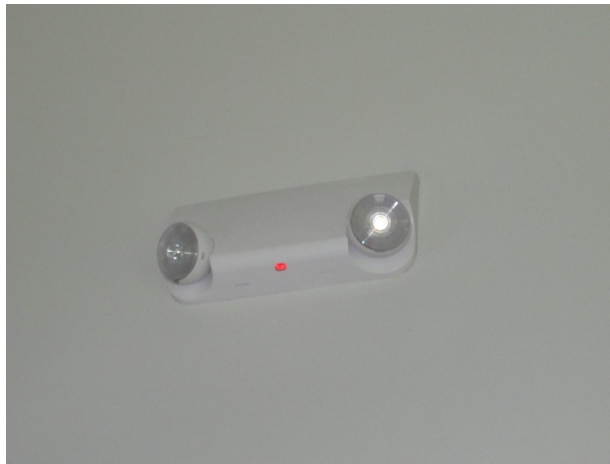
Emergency light fixture
