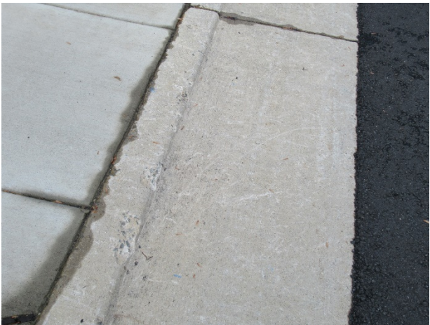
Concrete curb spall
