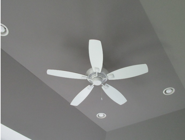
Clubhouse fan and interior recessed light fixtures
