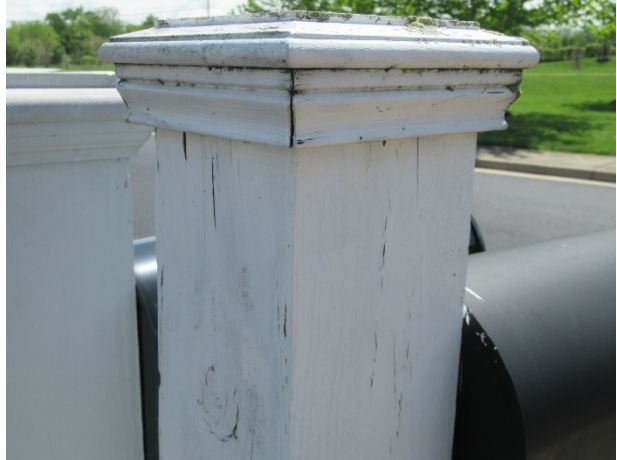
Paint finish and wood deterioration
