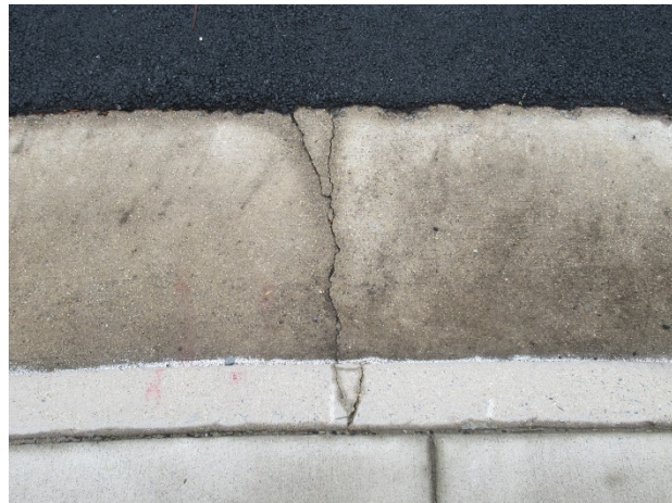
Concrete curb and gutter crack
