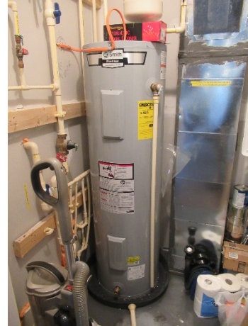
Clubhouse water heater
