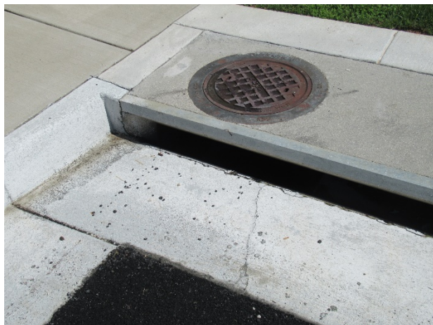
Concrete gutter crack adjacent to the catch basin structure
