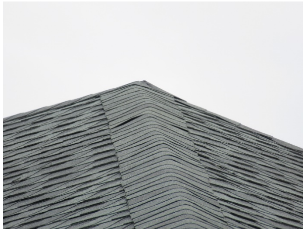
Isolated shingle lift at the ridge
