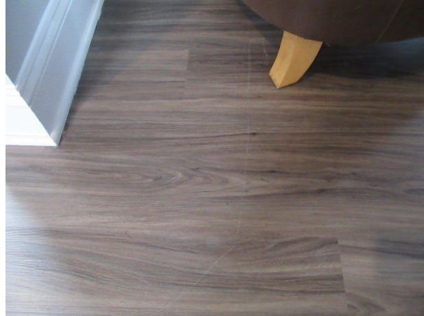
Tile floor scratch
