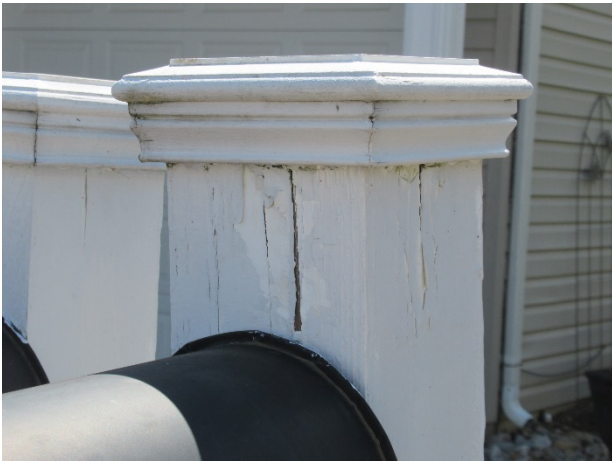
Paint finish and wood deterioration
