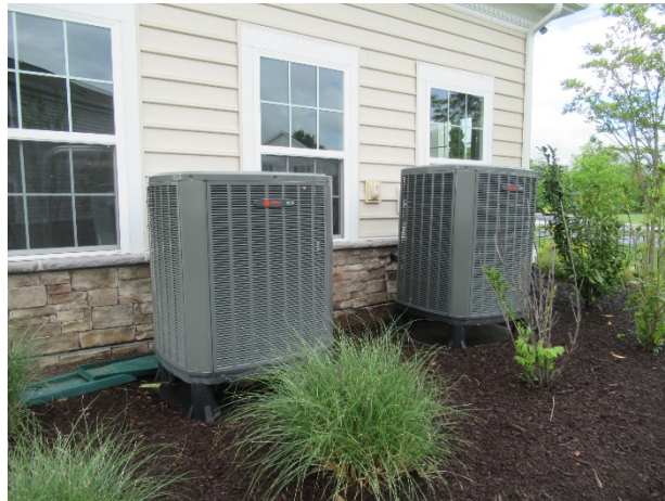
Split system condensing units
