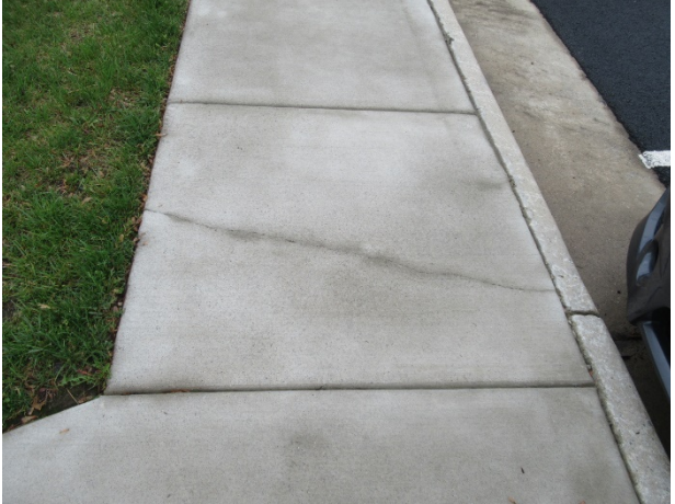
Concrete sidewalk crack
