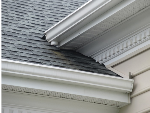
Missing downspout extension at the gutter discharge point
