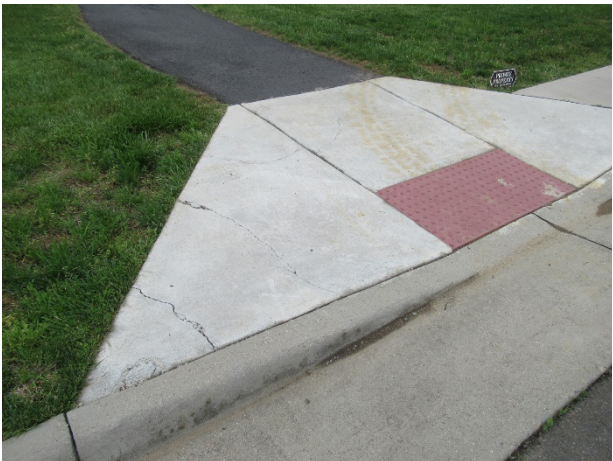
Concrete sidewalk crack
