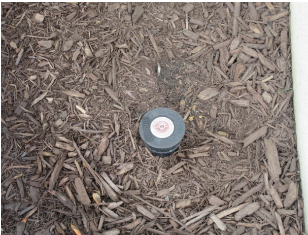
Clubhouse area irrigation system pop-up head
