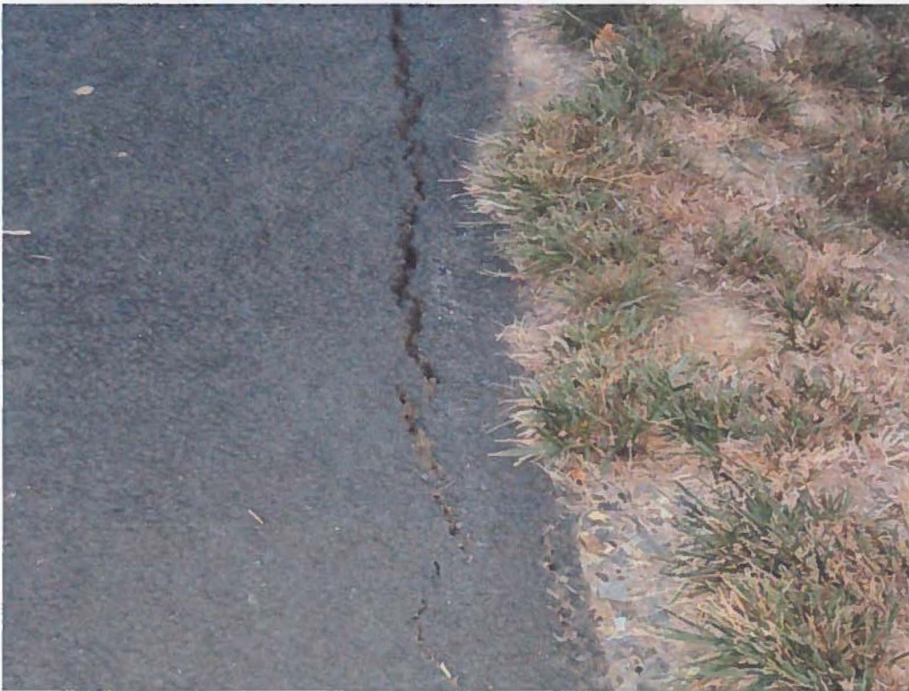
Photograph 10 - Cracked asphalt at foot path.
