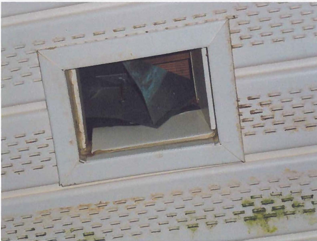
Photograph 8 – Loose dryer vent at balcony soffit.
