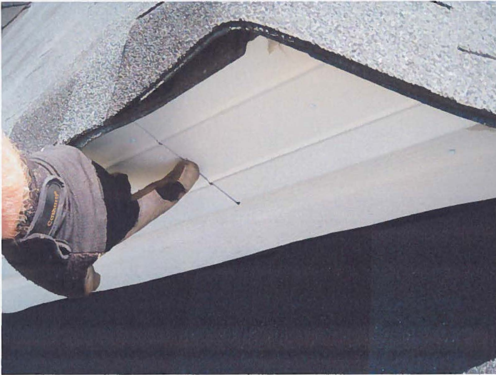
Photograph 1 - Improperly lapped trim cladding.
