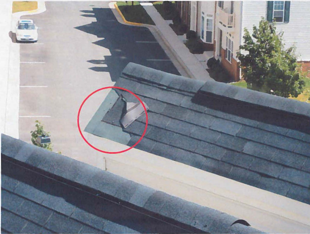
Photograph 5 – Wind damaged shingles.
