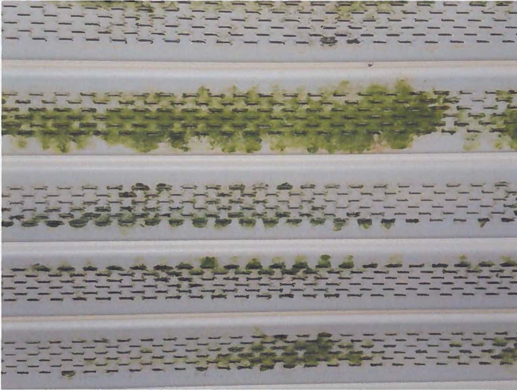
Photograph 9 - Algae staining on balcony soffit.
