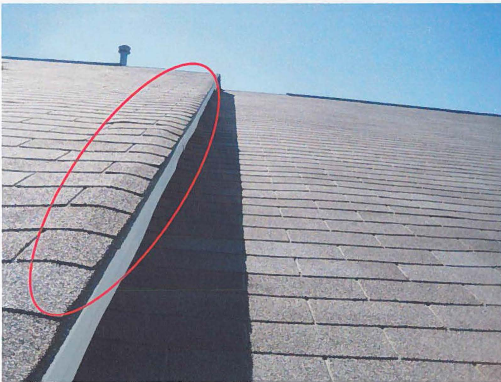
Photograph 6 – Shingles distorted due to excessive overhang.
