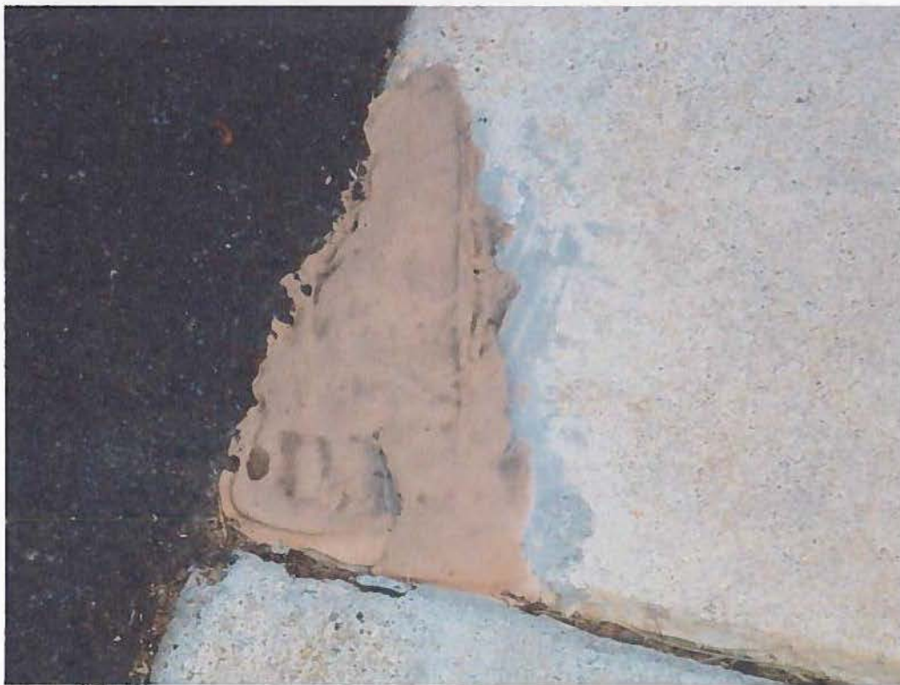
Photograph 12 – Substandard/unsightly repair at concrete sidewalk.
