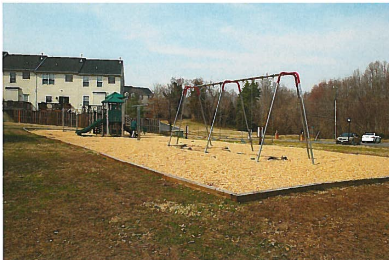
PHOTO #9 The upgraded replacement tot lot appears to be in good condition and should provide a long service life.
