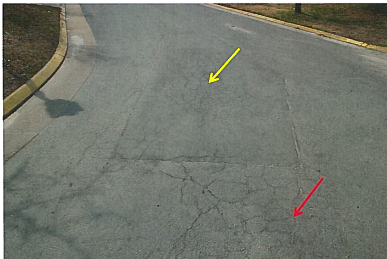
PHOTO #2 This area was repaired as recommended, but is now experiencing secondary deflection at the original full-depth repair patch (yellow) and radiating out beyond the original limits (red).
