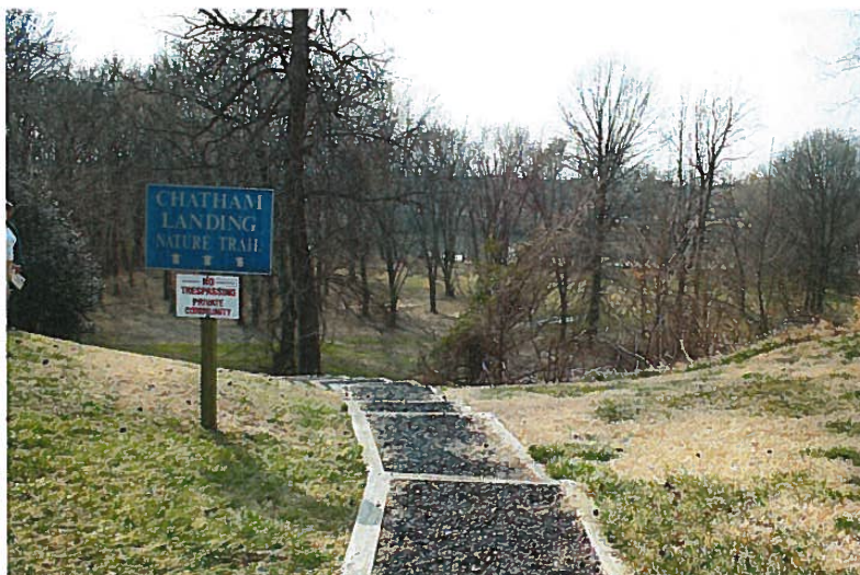
PHOTO #6 The gravel and wood timber steps and path is holding up well with a small amount of wood deterioration observed.
