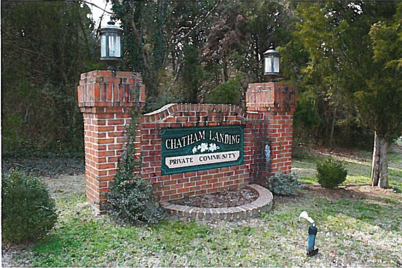
PHOTO #4 The monument appears to be in continuing good condition, albeit stained. Periodic acid cleaning of the masonry will renew appearance.
