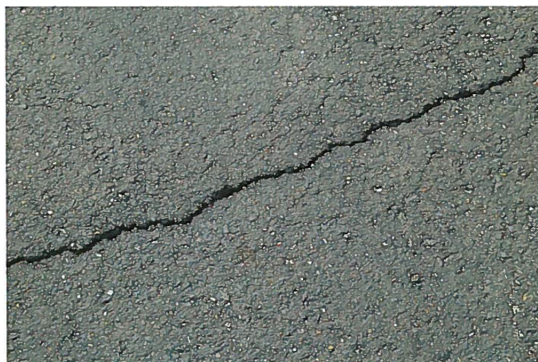
PHOTO #3 Random pavement cracking is now present to a limited degree. These cracks should be filled as part of the life-extension maintenance prior to the new application of seal coat.
