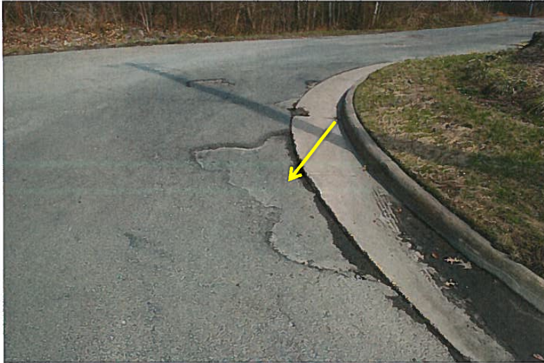
PHOTO #1 This area of pavement at the entrance has now delaminated from the base and requires repair to extend the service life.
