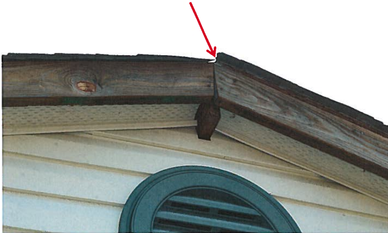
PHOTO #8 Minor repairs to the asphalt roofing shingles were not accomplished as suggested in 2003. This area should be repaired.
