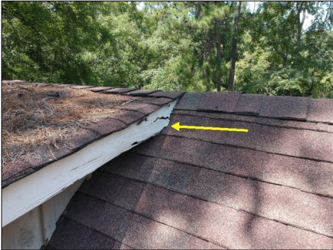
Replace the rotted fascia boards on the front & rear bonus room eaves.
