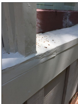
Replace the rotted window sill, sash and mulls at the rear left den triple window unit.
