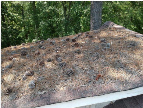
Have the heavy layer of pine straw removed from the bonus room roof & check for possible damage to the decking.
