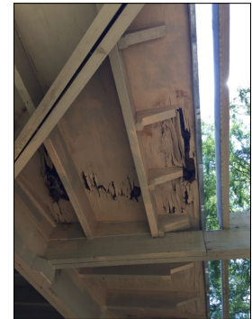
Replace all rotted roof decking and related framing damage at the rear porch roof.
