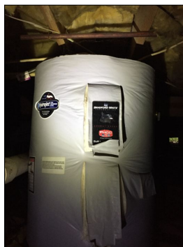
2014, Bradford white electric 40 gal water heater located in the crawl space.
