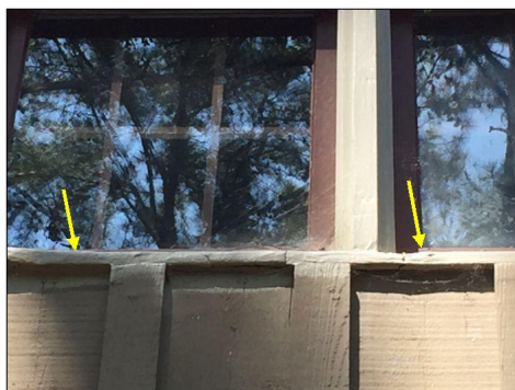
The window sill, sashes and mull are rotted at the upper left side, lower left side and front left side living room window units replace all damaged window componets as necessary.
