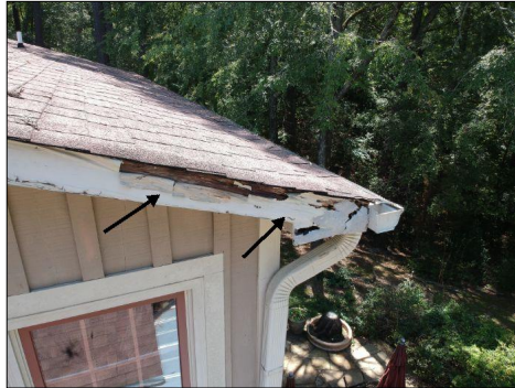
Replace the wood rot at the upper right side & rear eaves.
