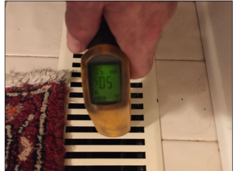
The AC system on the main level was cooling well during the inspection.
