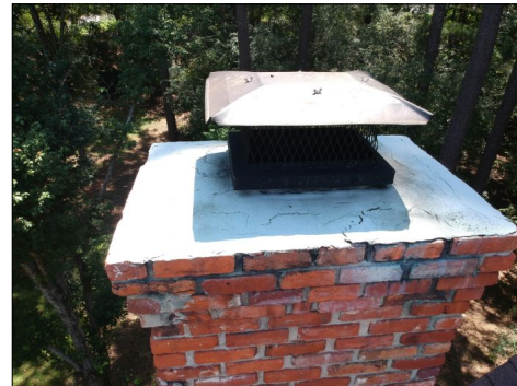
General minor brick deterioration noted on both chimneys which have been point tuckered & seem stable at this point, monitor for the need of further pointing up.
