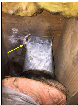
The AC vent boot should be insulated and caulked / sealed to the floor in the master bathroom.
