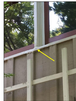
Replace the rotted window sill & mull at the front upper bonus room window.
