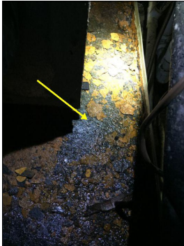
The over-flow pan under the HVAC unit in the attic is rust damaged and should be replaced.
