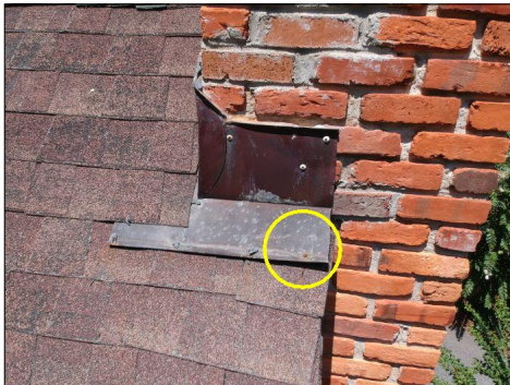
The chimney flashing fasteners should be re-caulked at both chimneys
