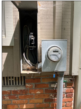
View of the 200 Amp electric service disconnect at the meter base.
