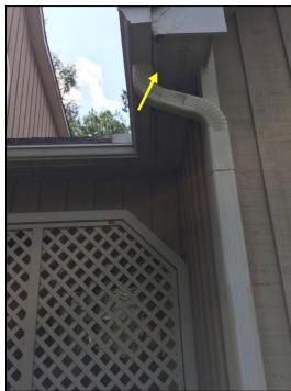
Replace water damaged fascia and soffit at the front left side of the master bedroom
