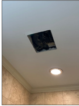
master bath exhaust fan cover is missing
