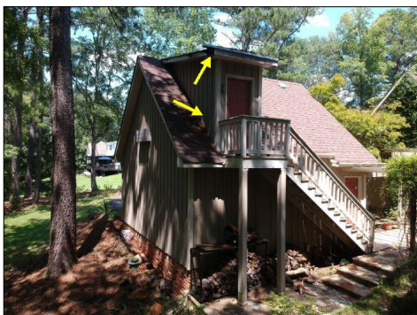
The sub-fascia board & possibly roof decking rot was observed as well as siding rot at the roof level on the upper rear bonus room outset area, replace all as needed.
