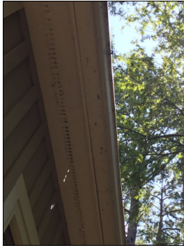
Replace the rusted out rear left gutter system.
