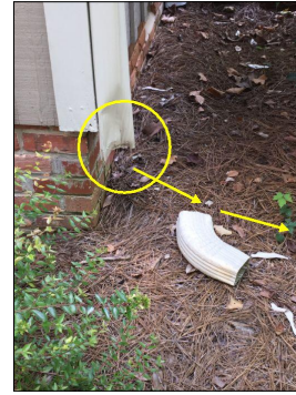
The front gutter down spouts should be extended to the left and right lower elevations of the lot using drain pipes to reduce water intrusion into the crawl space.
