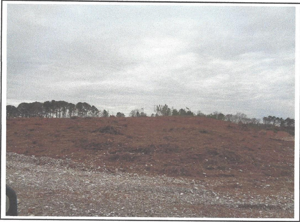
Photo 3 Eastern portion of Property, mound of dirt from trench construction, facing north.
