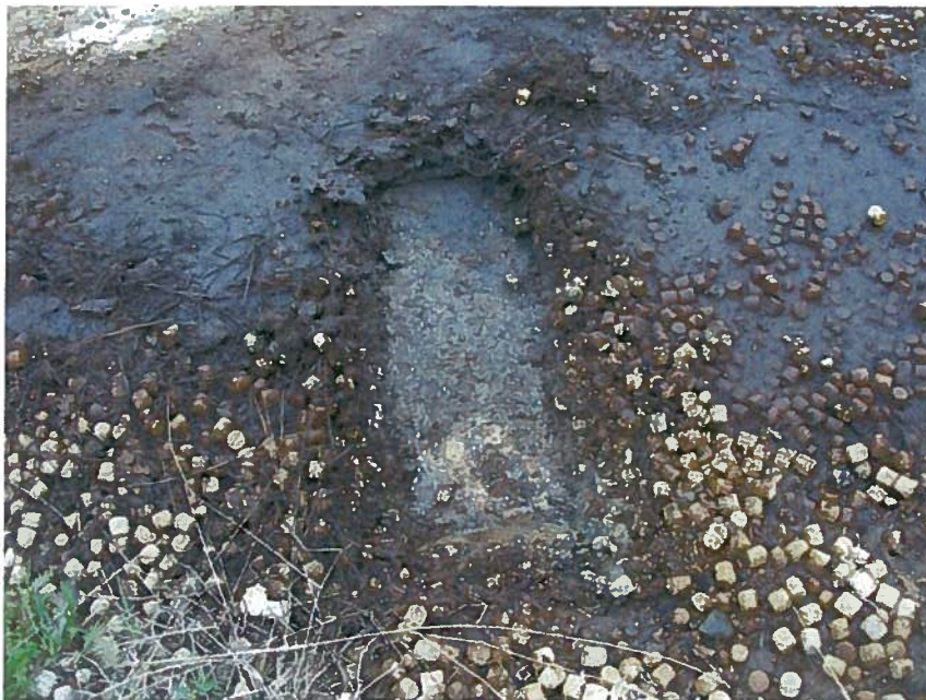
Photo 4: Close-up of asphalt underlying visually impacted soil at the former drum storage area.
