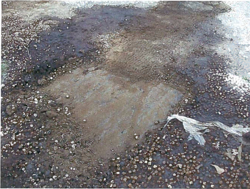
Photo 5: Excavation of visually impacted soil in progress at the former drum storage area.
