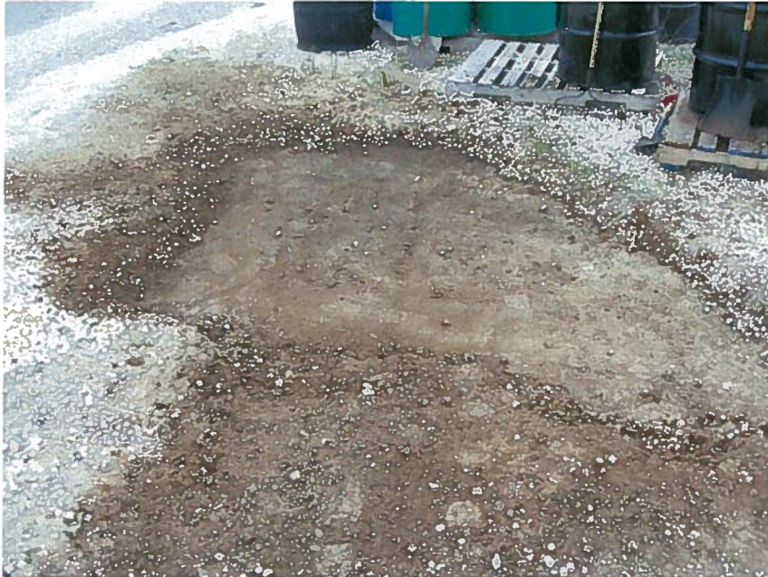
Photo 8: Close-up of visually impacted soil excavation at the former drum storage area complete (facing west).
