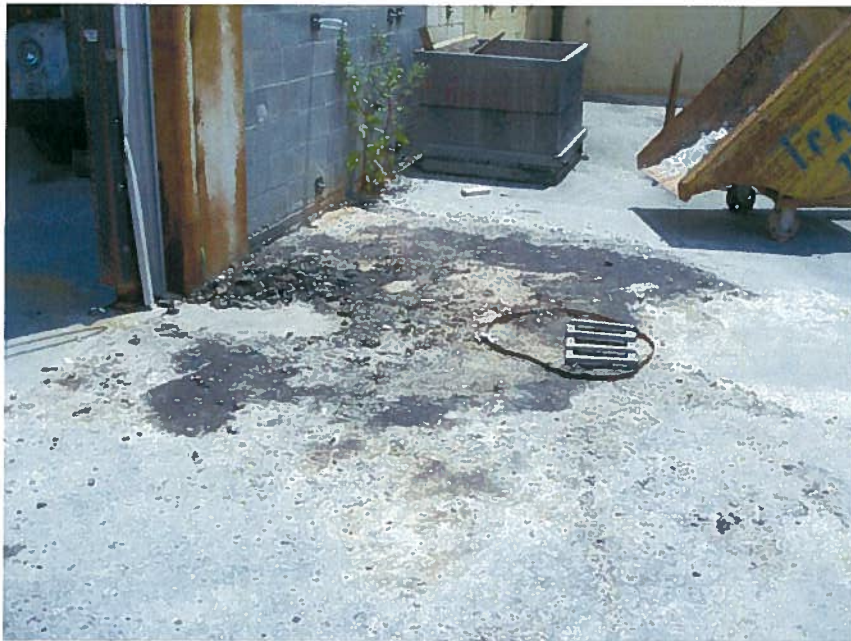
Photo 18: Visually impacted soil and asphalt behind the facility at boring location GP-6 (facing south).
