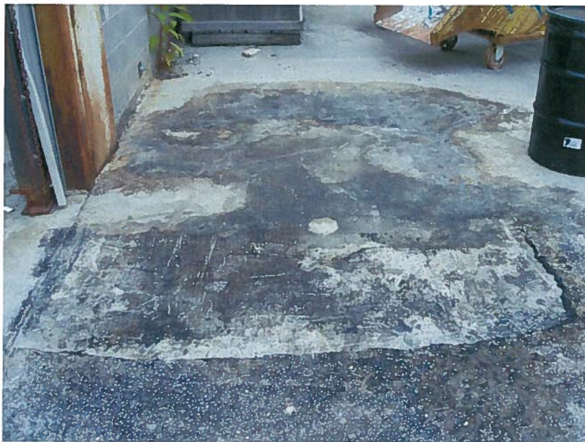
Photo 22: Close-up of visually impacted soil and asphalt excavation at the former drum storage area complete (facing south).
