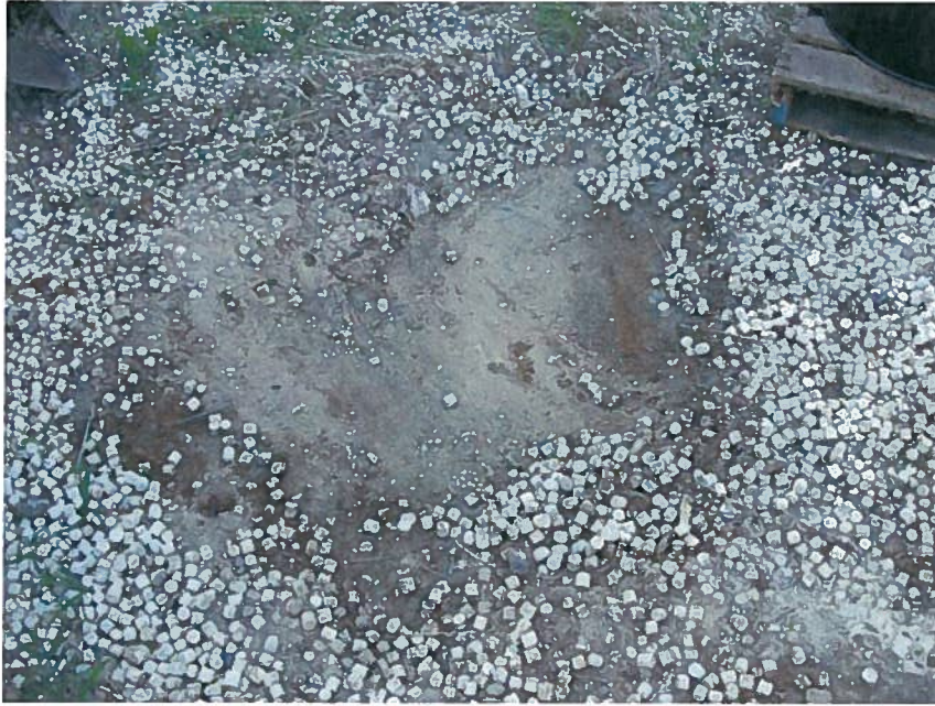
Photo 13: Excavation of a small area of visually impacted soil at the former drum storage area complete.
