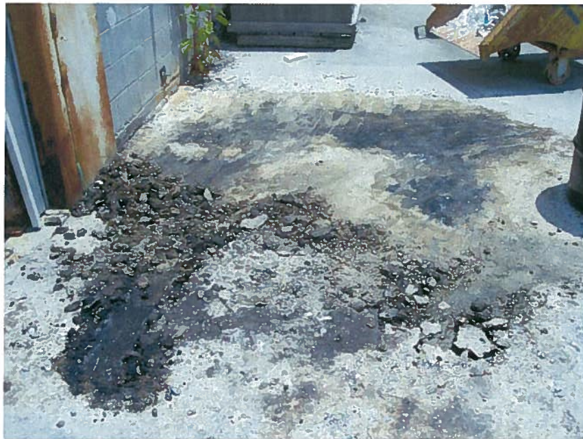
Photo 20: Excavation of visually impacted soil and asphalt in progress behind the facility at boring location GP-6.
