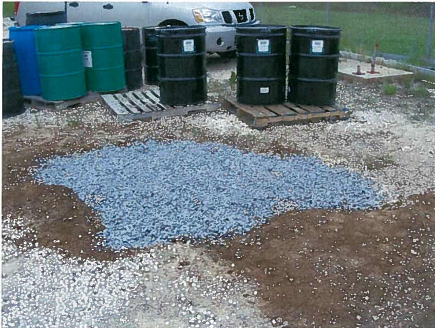
Photo 10: Gravel backfill in the visually impacted soil excavation at the former drum storage area (facing west).
