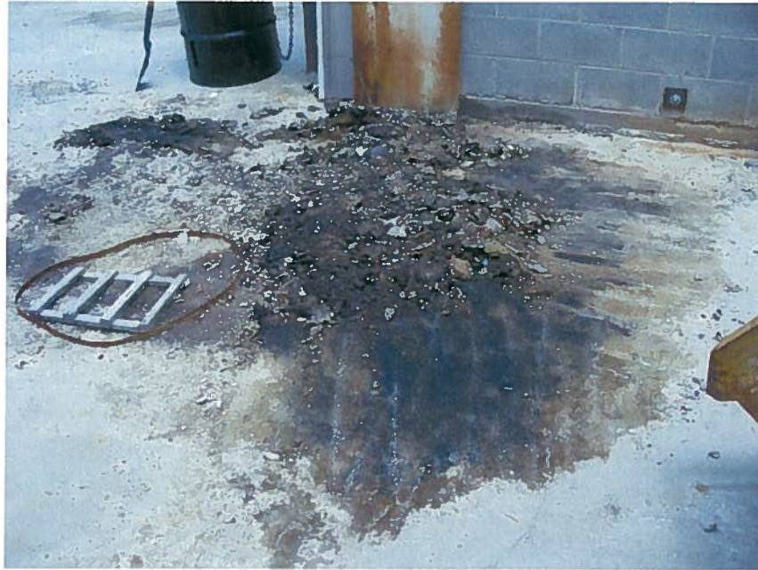
Photo 19: Excavation of visually impacted soil and asphalt in progress behind the facility at boring location GP-6.
