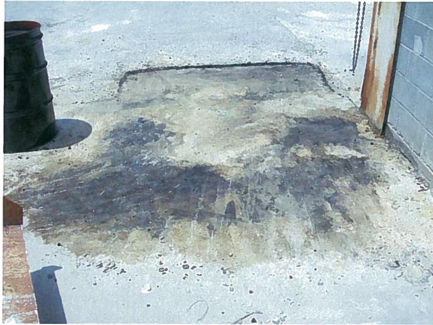
Photo 21: Close-up of visually impacted soil and asphalt excavation at the former drum storage area complete (facing north).
