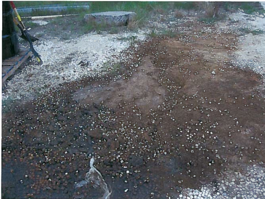
Photo 6: Excavation of visually impacted soil in progress at the former drum storage area.
