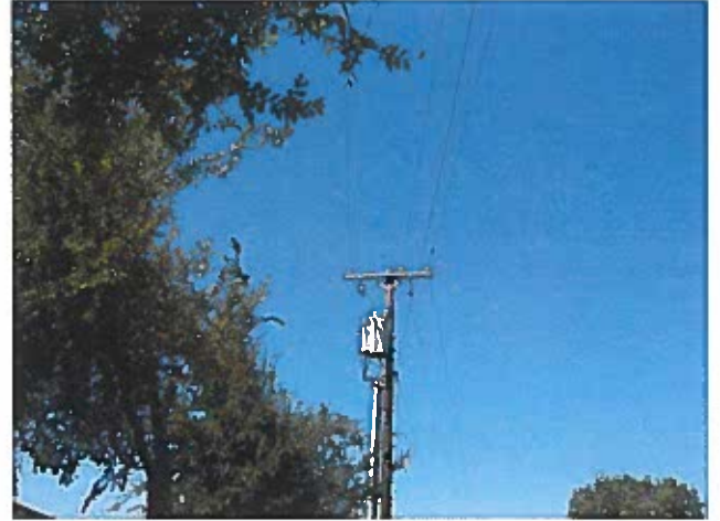
Photo #14: Pole-Mounted Transformers on North Border
