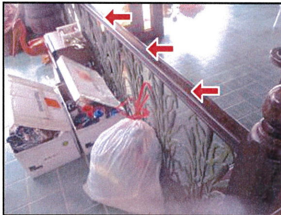
4.3 Picture 1 Guard railing in sun room was very loose
