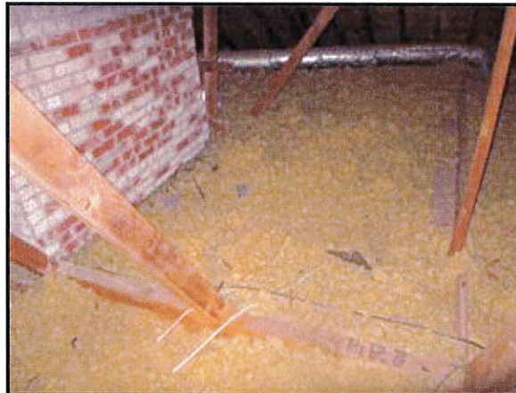
9.0 Picture 1 View of attic insulation
