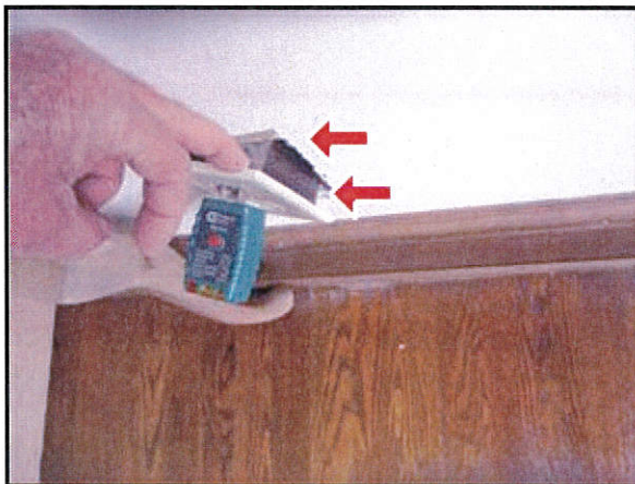
7.3 Picture 3 Electrical box at upstairs hallway was not properly secured inside wall as required .
