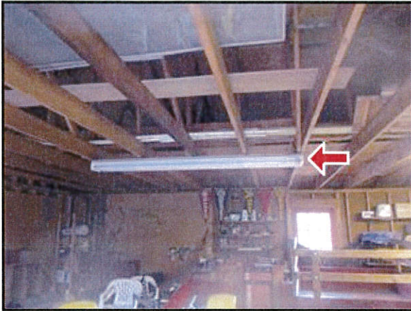
7.3 Picture 5 One of the light fixtures located inside the detached shop building was inoperable .
