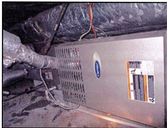
8.0 Picture 3 Furnace / air handler located in crawl space
