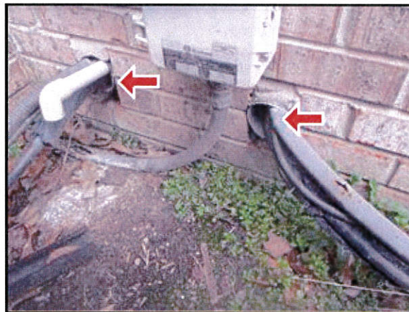
2.0 Picture 5 Pipe and wire penetrations through exterior walls were not sealed .
