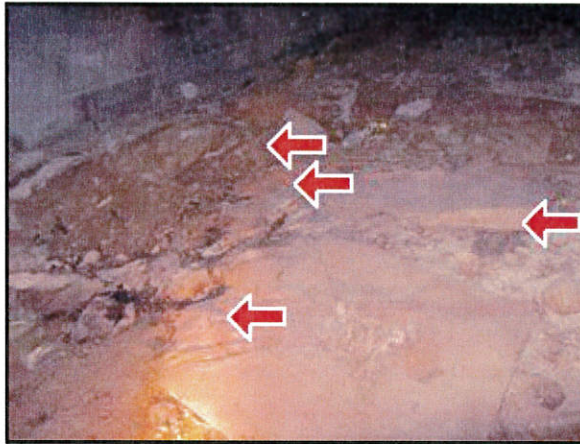
9.2 Picture 1 Cellulose debris in crawl space . No vapor barrier installed .
