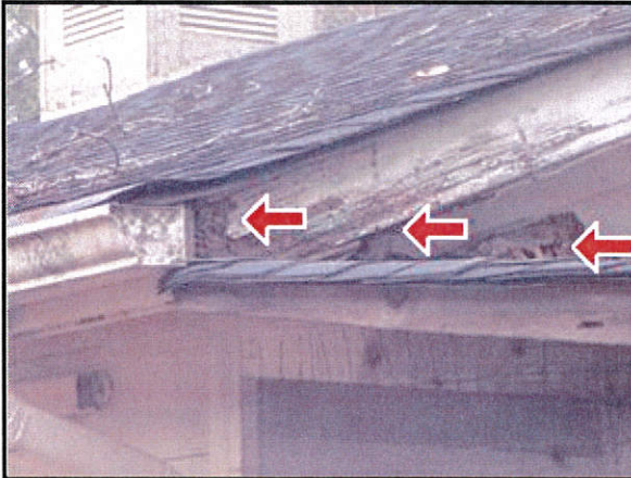
2.6 Picture 1 Fascias and soffits were water damaged and deteriorated at various locations around the detached shop building .
