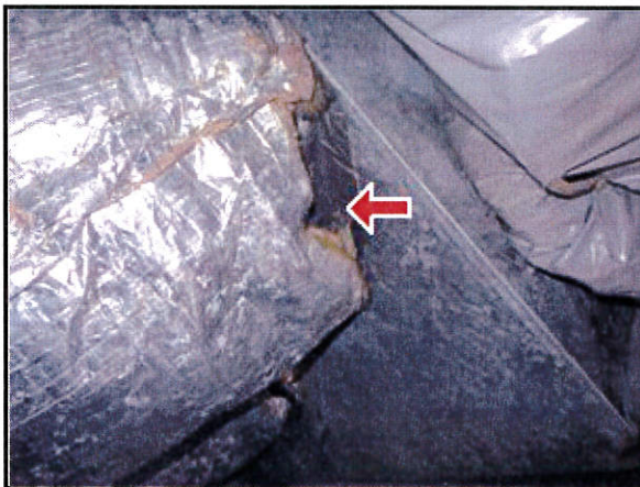
8.3 Picture 1 HVAC duct work was not properly sealed to air handler plenums
