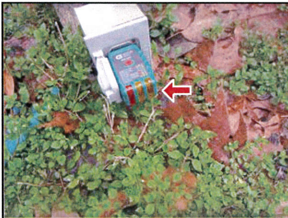
7.3 Picture 7 Receptacle located at ground level at end of retaining wall in rear yard was not operable .
