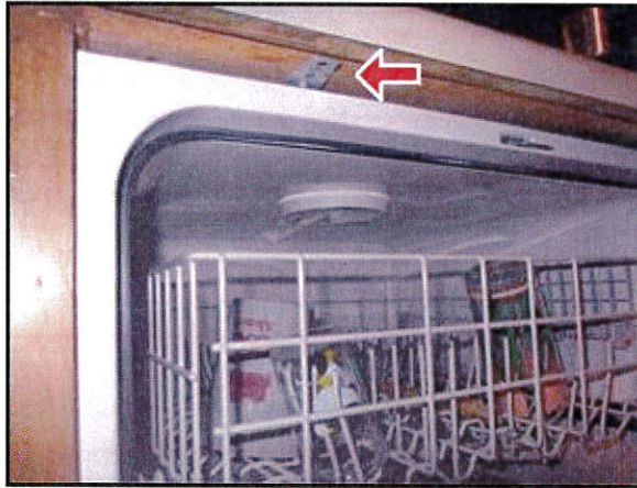
10.0 Picture 1 Dishwasher not secured to cabinet
