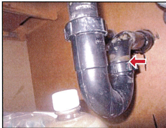
6.0 Picture 1 Leak notec at left master sink drain .
