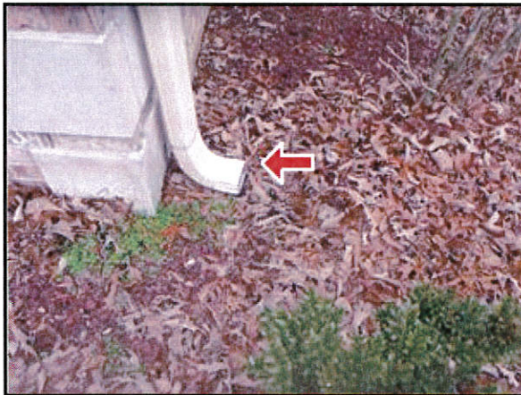
1.3 Picture 1 Downspouts terminate too close to the house
