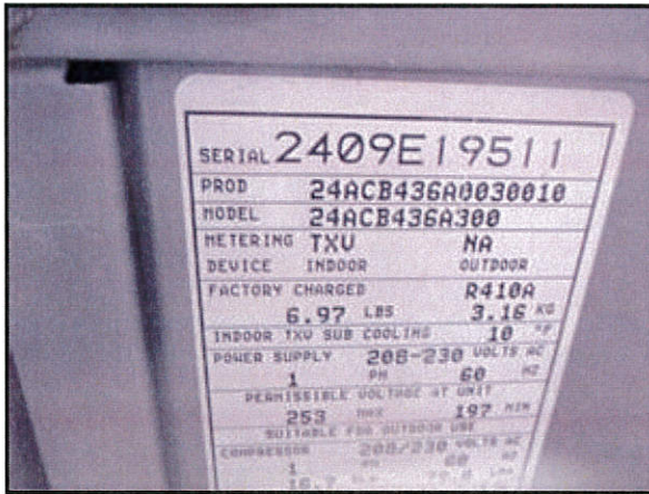
8.8 Picture 3 Air conditioning manufacturers data plate
