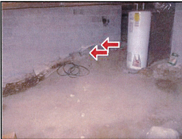
5.0 Picture 1 Old , dry moisture stains noted on crawl space foundation block walls at various locations .
