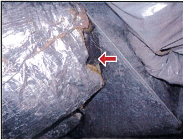
8.3 Picture 1 HVAC duct work was not properly sealed to air handler plenums
