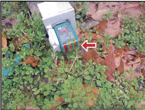
7.3 Picture 7 Receptacle located at ground level at end of retaining wall in rear yard was not operable .
