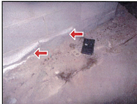
5.0 Picture 2 Old , dry moisture stains on block foundation walls in crawl space
