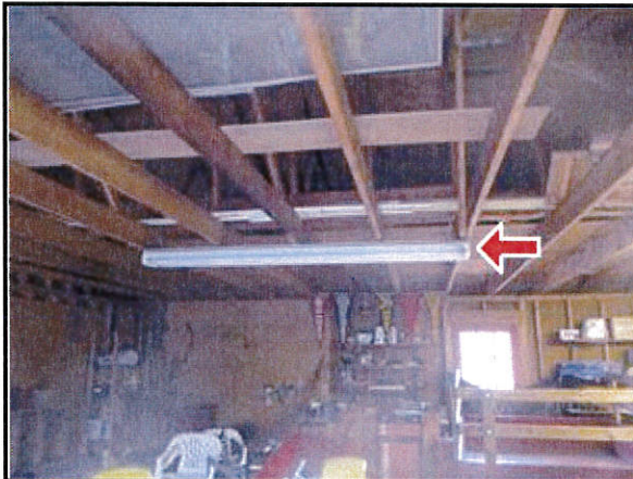
7.3 Picture 5 One of the light fixtures located inside the detached shop building was inoperable .
