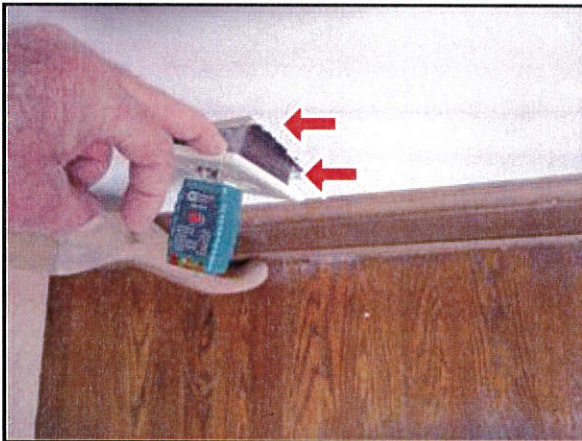
7.3 Picture 3 Electrical box at upstairs hallway was not properly secured inside wall as required .
