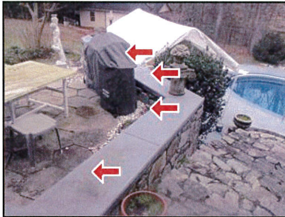
2.3 Picture 5 There was no guard railing installed at rear patio / retaining wall .
