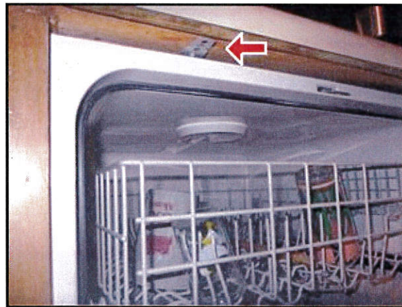
10.0 Picture 1 Dishwasher not secured to cabinet
