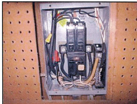
7.2 Picture 4 Sub panel in the detached shop building with cover removed
