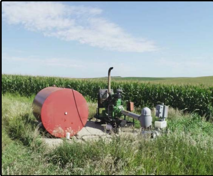
Power Unit, Well, Diesel Tank
