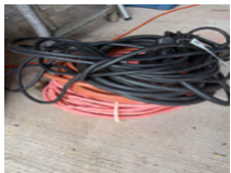
#80 • Three electrical cords
