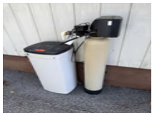
#140 • Water treatment system
