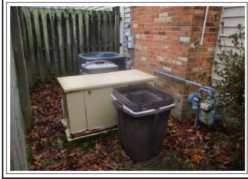
view of whole house generator
