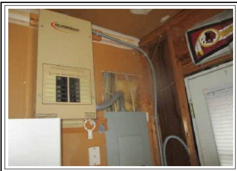
view of panel box and generator switch
