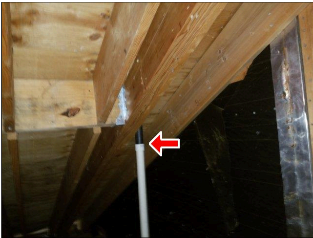
12.2 DRAIN / WASTE PIPING Photo 1
