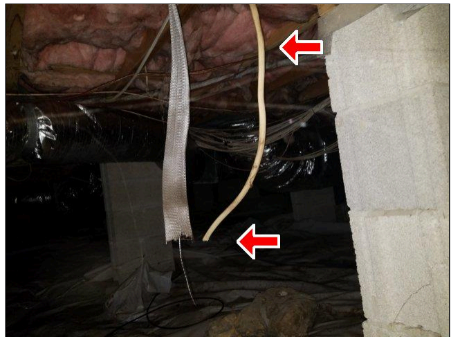
10.6 WIRING / CONDUCTORS Photo 2
