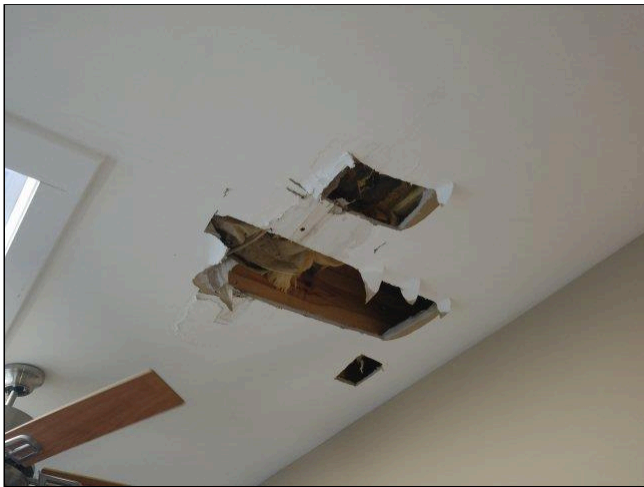
1.3(1) EXPOSED FLASHING Photo 1
