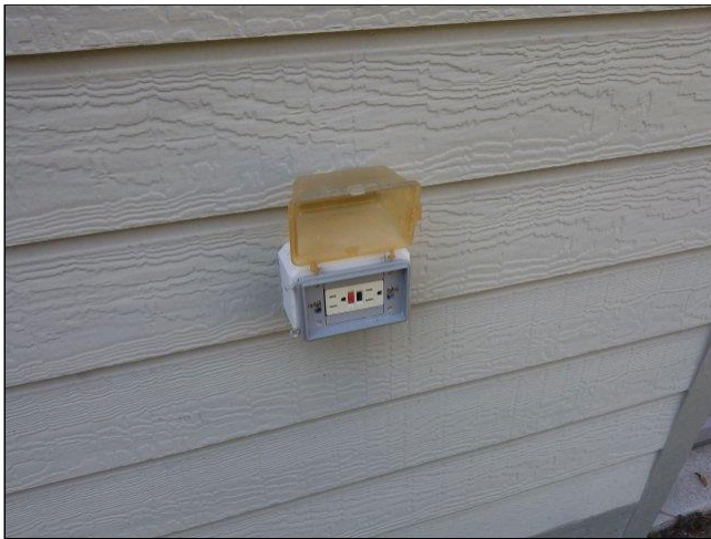
4.10.A ELECTRIC / GFCI Photo 1
