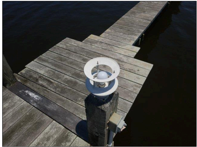
2.10 ELECTRIC / GFCI Photo 1
