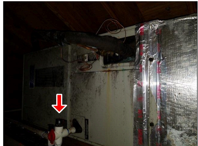
11.3(2) CONDENSATE PROVISIONS Photo 1
