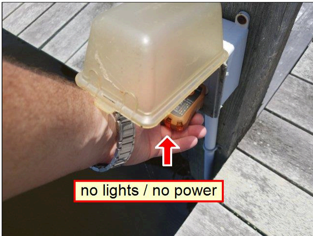
2.10 ELECTRIC / GFCI Photo 2
