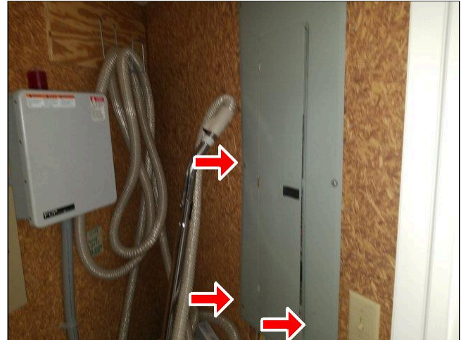
10.3(1) DISTRIBUTION PANEL(S) Photo 1
