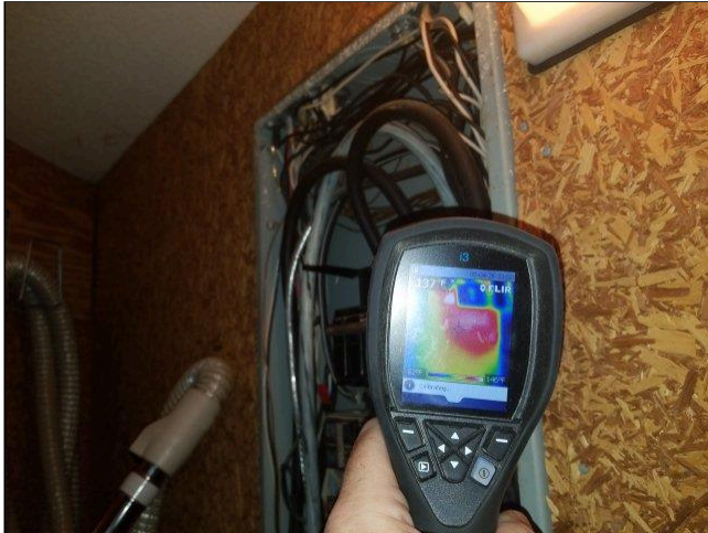
10.2 MAIN DISCONNECT(S) Photo 1
