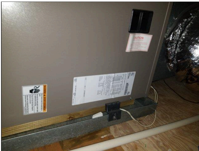
4.11.A HEATING & COOLING Photo 2
