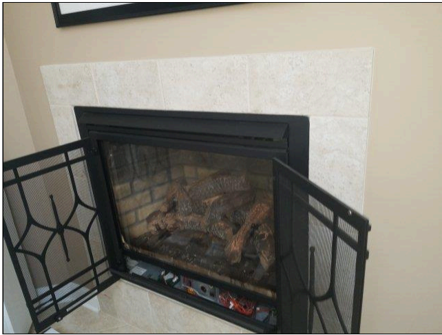
8.10(1) FIREPLACE GAS BURNERS Photo 1
