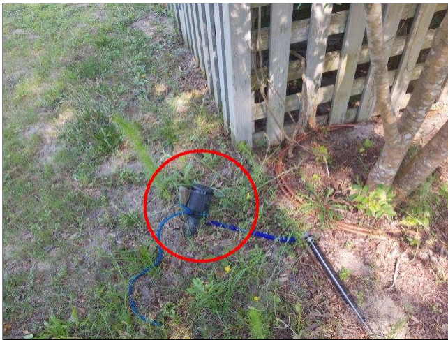
3.7 LAWN IRRIGATION SYSTEM Photo 1
