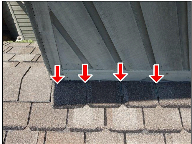
1.3(2) EXPOSED FLASHING Photo 1
