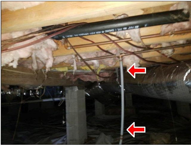
12.0 WATER PIPING Photo 1
