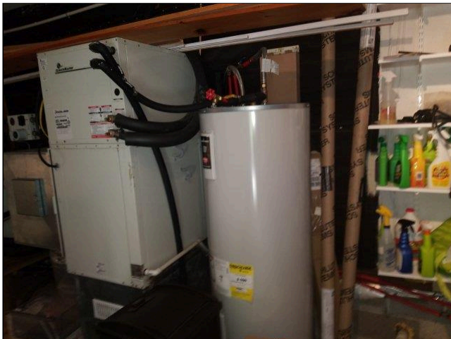
13.0 WATER HEATER(S) Photo 1
