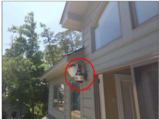
2.10 ELECTRIC / GFCI Photo 3
