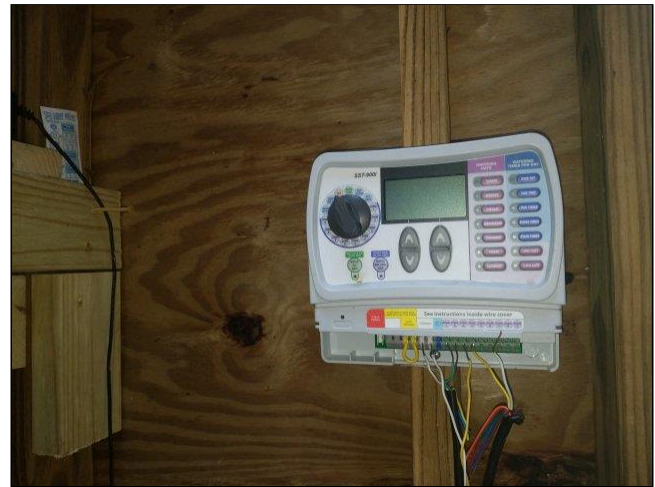
3.7 LAWN IRRIGATION SYSTEM Photo 2
