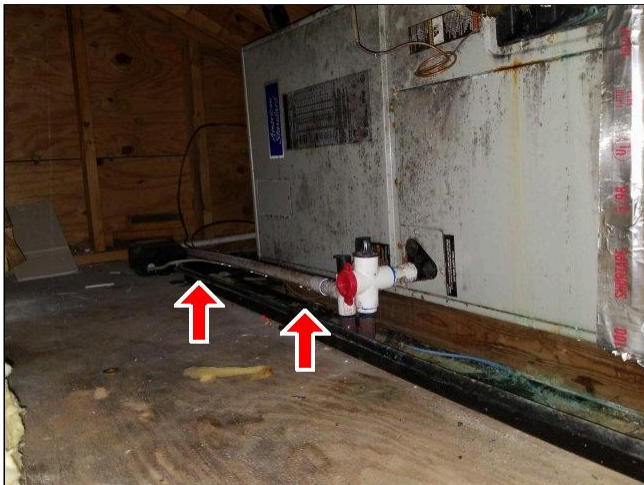
11.3(1) CONDENSATE PROVISIONS Photo 1
