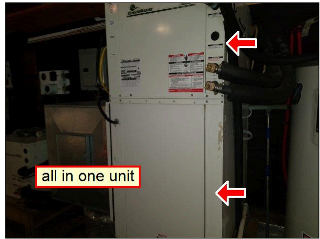
11.0 HEAT PUMP SYSTEM(S) Photo 2
