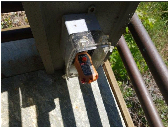
2.10 ELECTRIC / GFCI Photo 4
