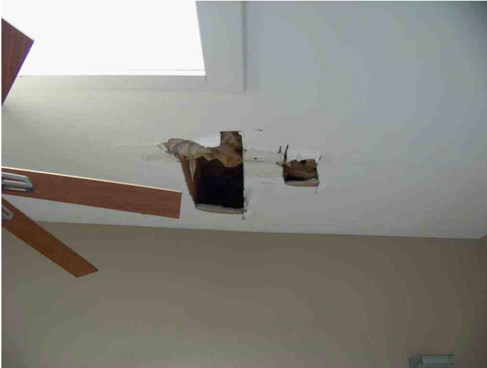
Sheetrock Damage in the Ceiling to the First Floor Sunroom
