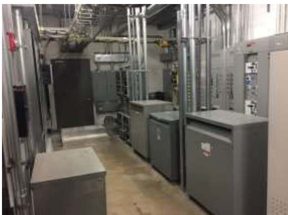
Un-cooled electrical room (Photo Taken on July 20, 2017)
