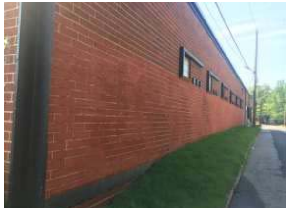
Looking southerly on Curran Street on west-side of Bldg. (Photo Taken on July 20, 2017)
