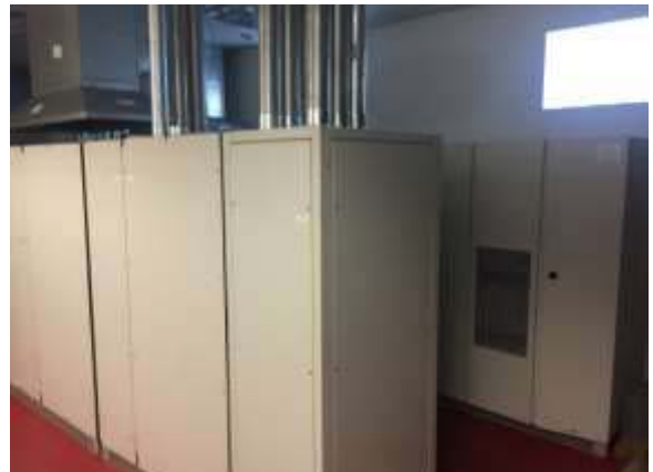
UPS room (Photo Taken on July 20, 2017)
