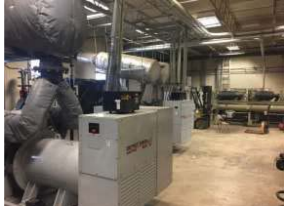
Warehouse finish space- chiller plant room (Photo Taken on July 20, 2017)
