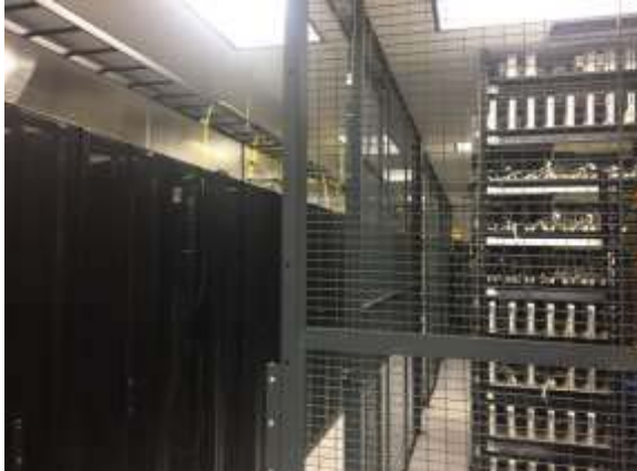
Raised-floor data center space (Photo Taken on July 20, 2017)
