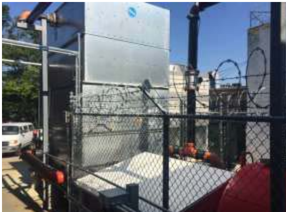
2016 Chiller Plant installed on north of building (Photo Taken on July 20, 2017)
