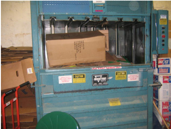
Photo #7: Cardboard bailer located within the warehouse
