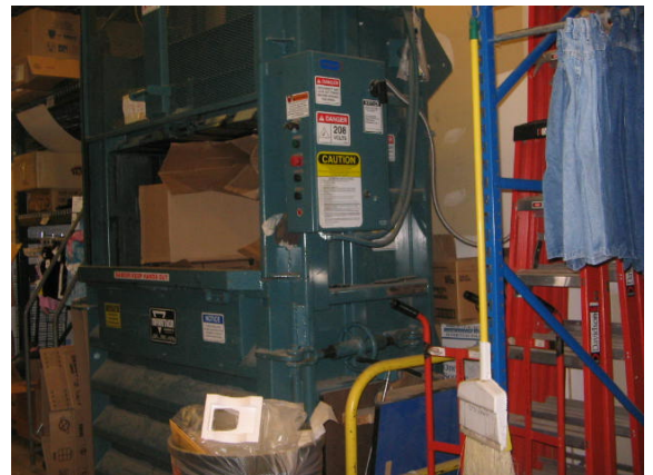
Photo #6: Cardboard compactor
