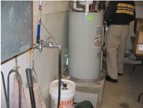
Photo #1: Water heater in maintenance room
