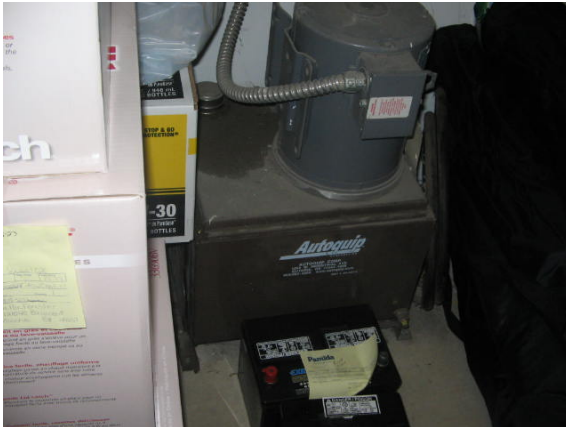
Photo #7: Hydraulics reservoir for loading dock lift
