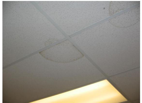
Photo #4: Water damage to ceiling in main retail area
