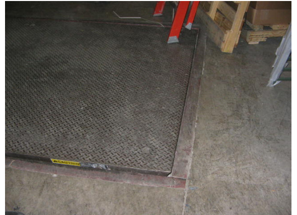
Photo #8: Loading dock lift
