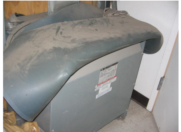
Photo #2: Dry secondary step-down transformer in maintenance room
