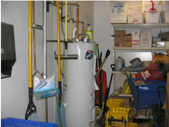
Photo #1: Water heater in maintenance room
