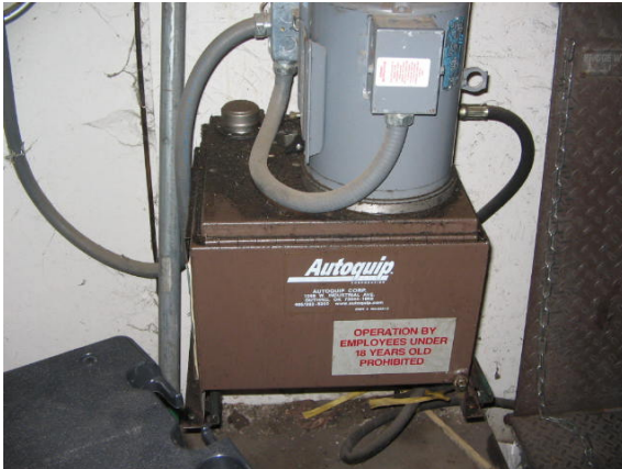
Photo #7: Hydraulics reservoir for loading dock lift
