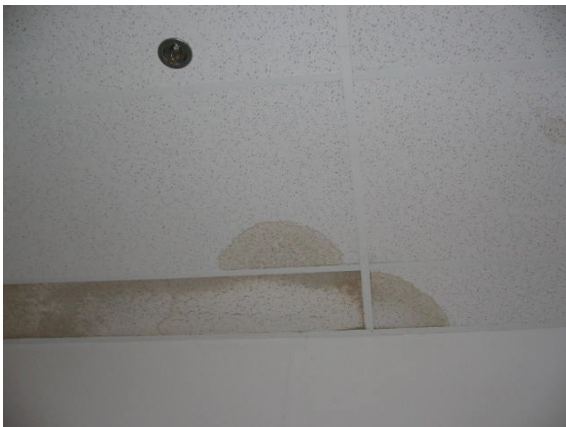
Photo #5: Water damage to ceiling in lay-a-way room
