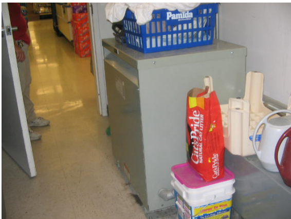
Photo #11: Dry type step down transformer in maintenance room
