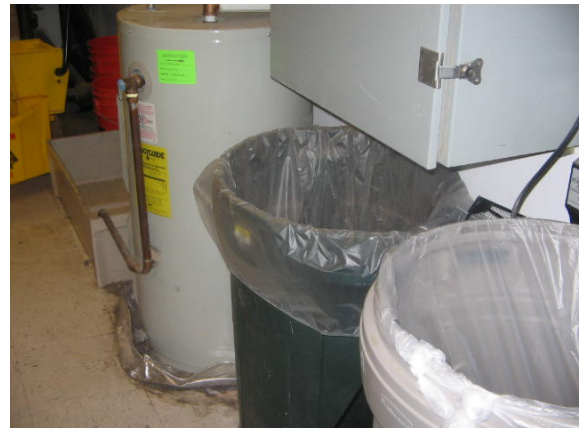
Photo #10: Water heater in maintenance room
