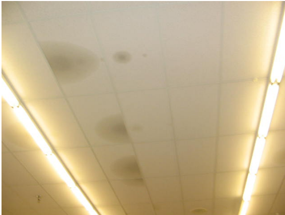
Photo #13: Visible suspect mold on ceiling in main retail area
