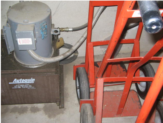
Photo #7: Hydraulics reservoir for loading dock lift
