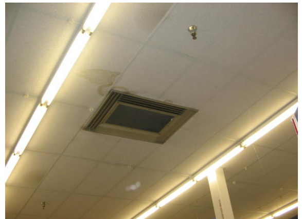
Photo #12: Water damage on ceiling in main retail area
