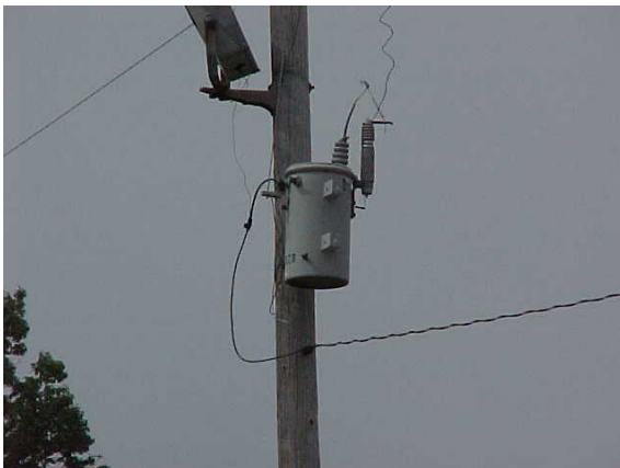
Photo #5: Pole-mounted transformer
