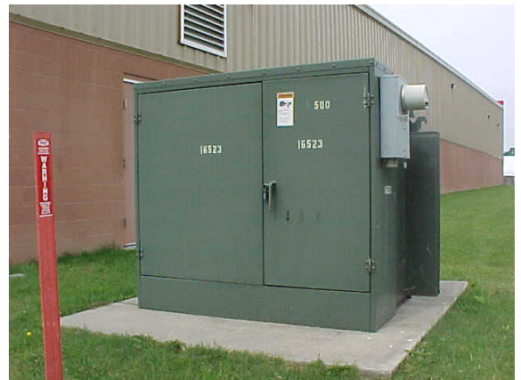
Photo #6: Pad-mounted transformer
