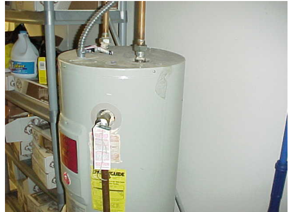
Photo #8: Electric water heater
