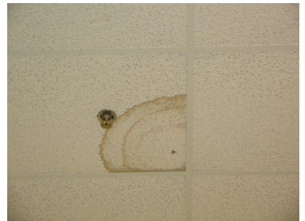
Photo #16: Water damage in retail area
