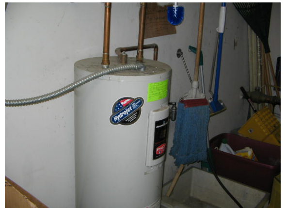
Photo #12: Water heater
