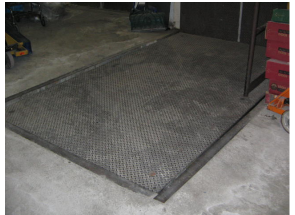
Photo #10: Hydraulic freight lift
