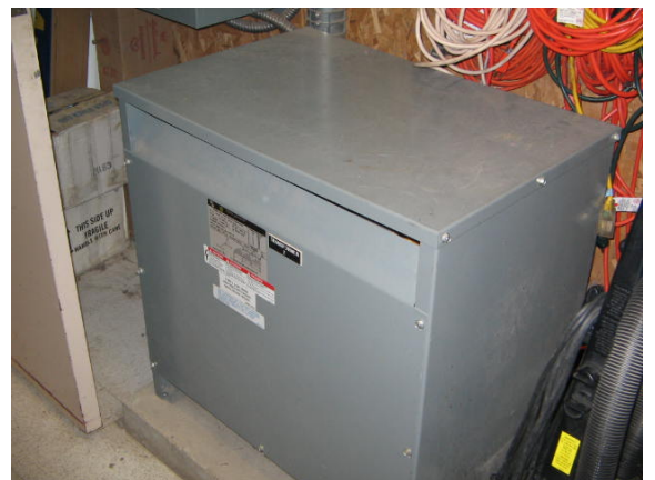
Photo #8: Dry transformer
