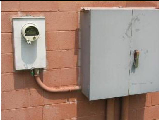
Photo #9: Electric meter. Section 5.1
