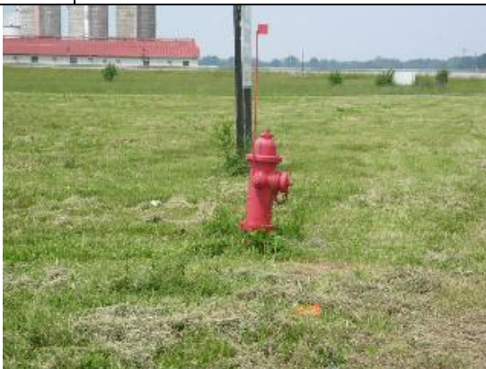
Photo #15: Fire hydrant. Section 7.6
