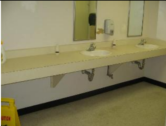
Photo #23: Tenant restroom vanities. Section 8.1
