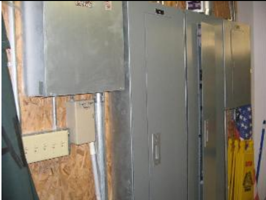
Photo #11: Circuit breaker panels. Section 5.1
