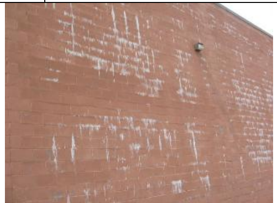
Photo #28: CMU wall efflorescence. Section 6.4
