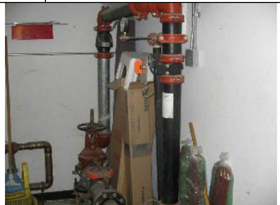
Photo #16: Sprinkler riser. Section 7.6
