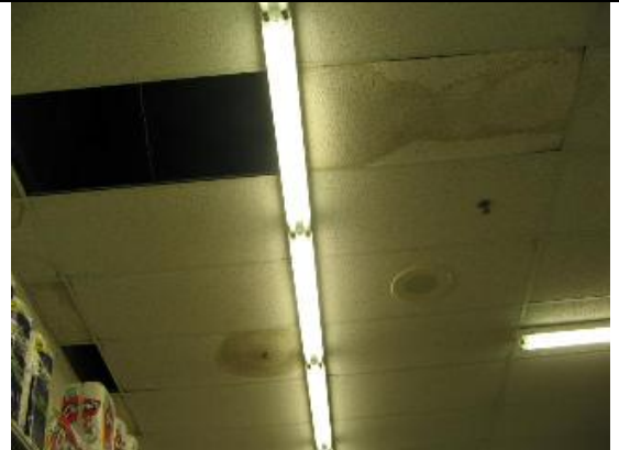
Photo #30: Damaged ceiling tiles. Section 8.1
