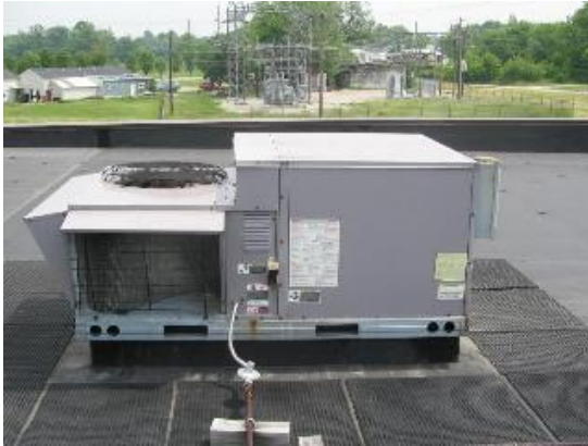
Photo #13: Rooftop unit. Section 7.1
