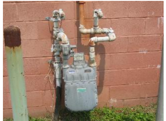
Photo #8: Gas meter and regulator. Section 5.1
