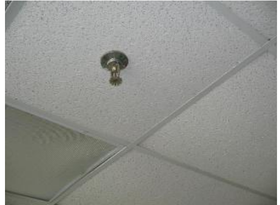
Photo #14: Sprinkler head. Section 7.6
