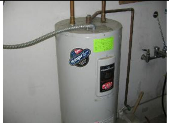
Photo #12: Water heater. Section 7.2
