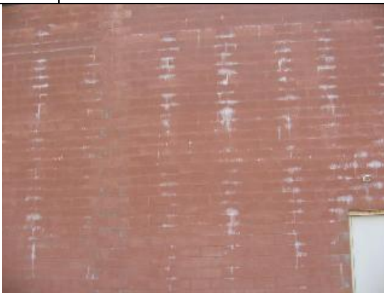
Photo #27: CMU wall efflorescence. Section 6.4
