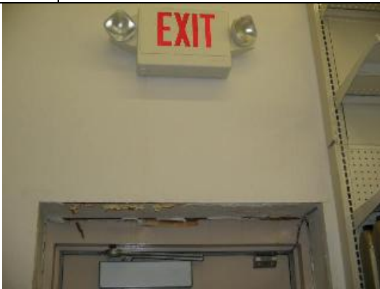
Photo #17: Emergency light and exit sign above drywall damaged door. Section 7.6
