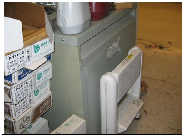
Photo #8: Dry type transformer
