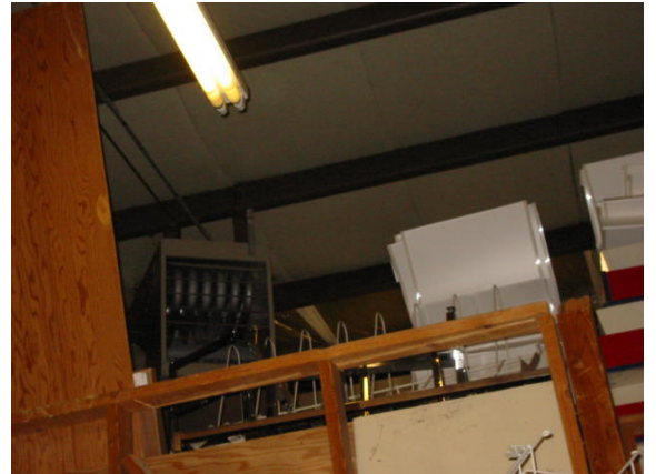
Photo #8: Natural gas-fired space heater in warehouse
