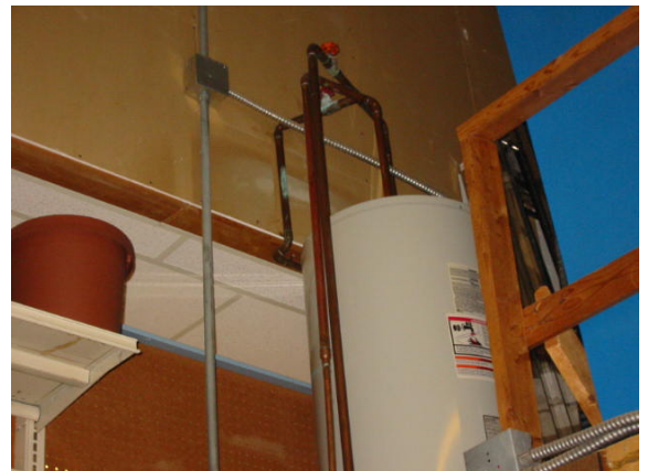
Photo #6: Natural gas-fired hot water heater
