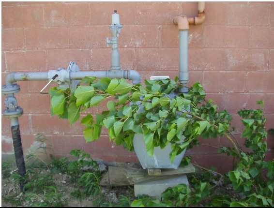
Photo #7: Natural gas meter
