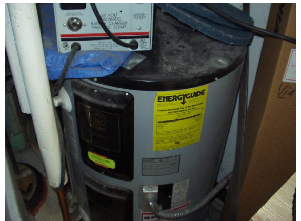
Photo #10: Electric water heater
