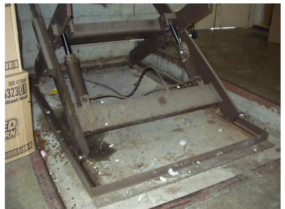
Photo #12: Dock lift
