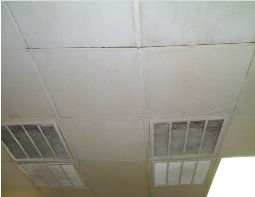
Photograph depicts water damaged/sagging ceiling tiles in the kitchen. According to Mr. Everett, when it rains, it leaks in the kitchen and front entrance. Roofers have been contracted but cannot find source of leak.
