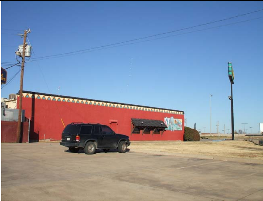
Photograph depicts the south side of the building, view facing northeast. Photograph depicts the pole-mounted transformers.
