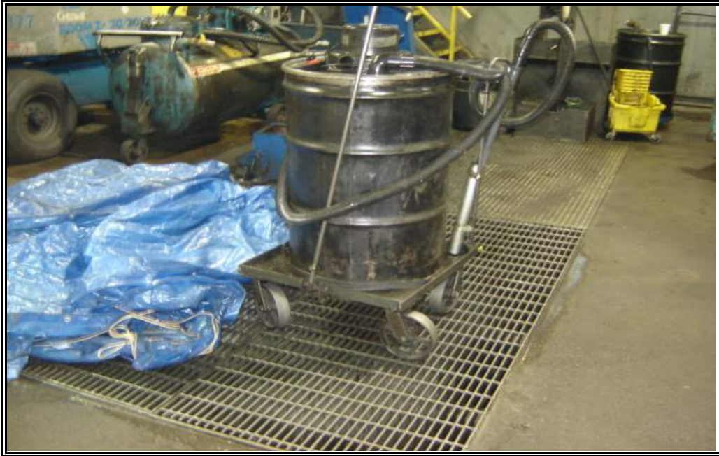
View of the waste coolant and oil separator (below grade containment) in the oil/chip room of Plant #1.
