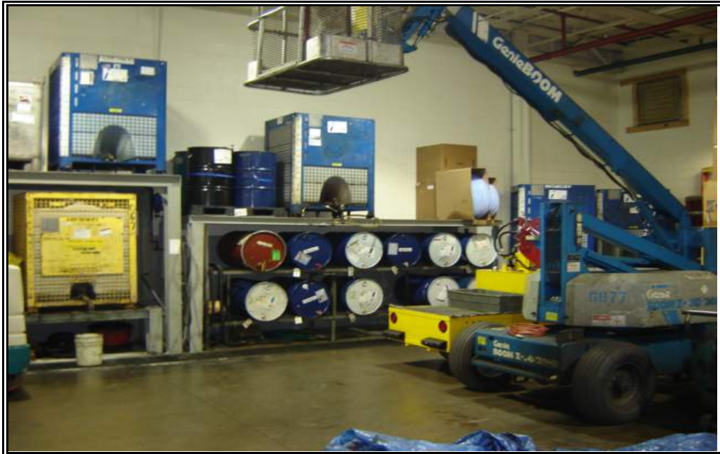
View of the drum and AST storage located within the oil/chip room of Plant #1.
