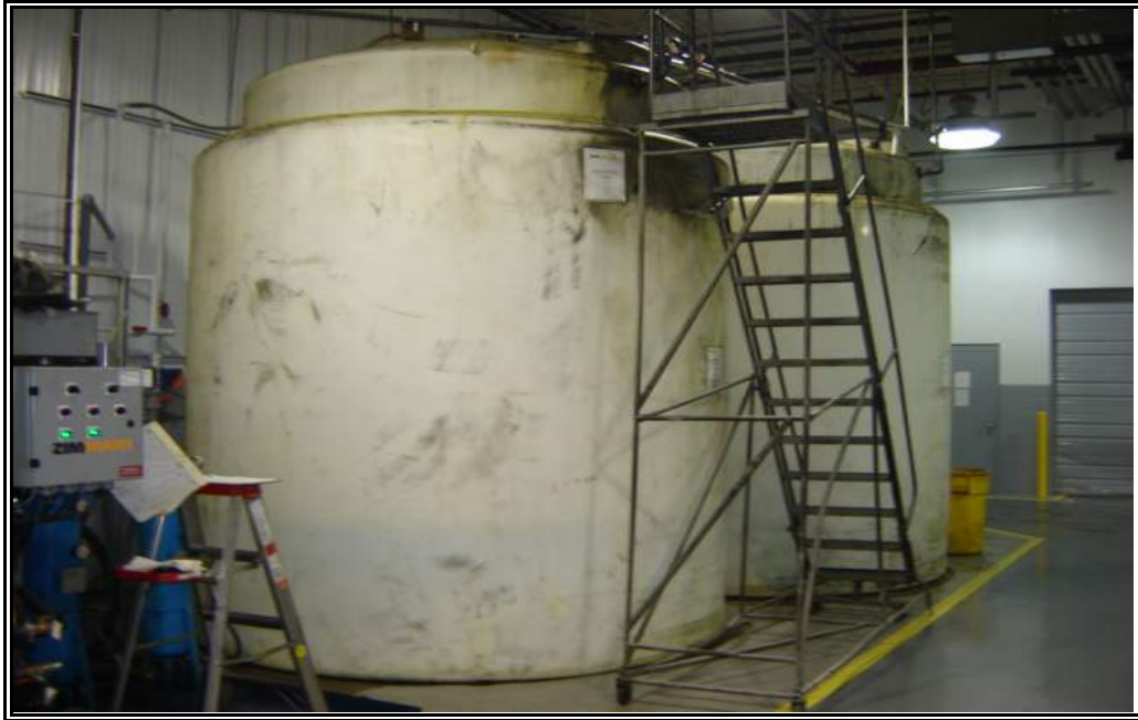
View of the ASTs used as part of the coolant recycling system, located in Plant #1.
