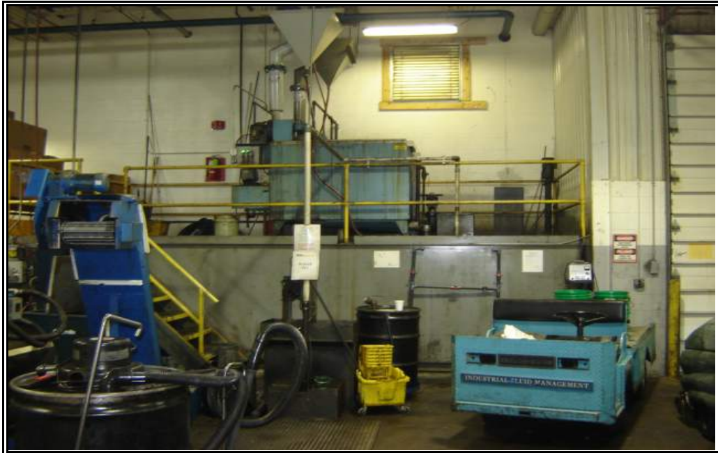
View of the waste coolant separator system in the oil/chip room of Plant #1.
