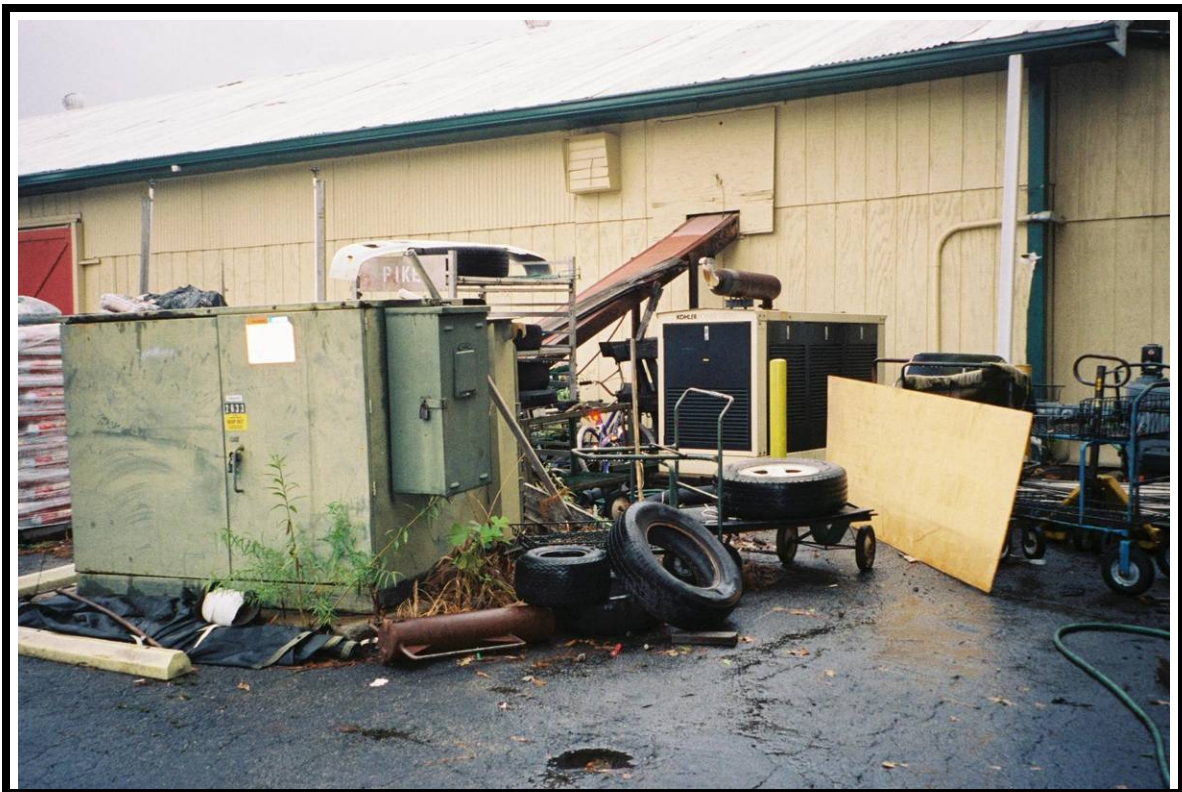
4. View of the pad-mounted transformer and the backup generator adjacent to the maintenance shop area.
