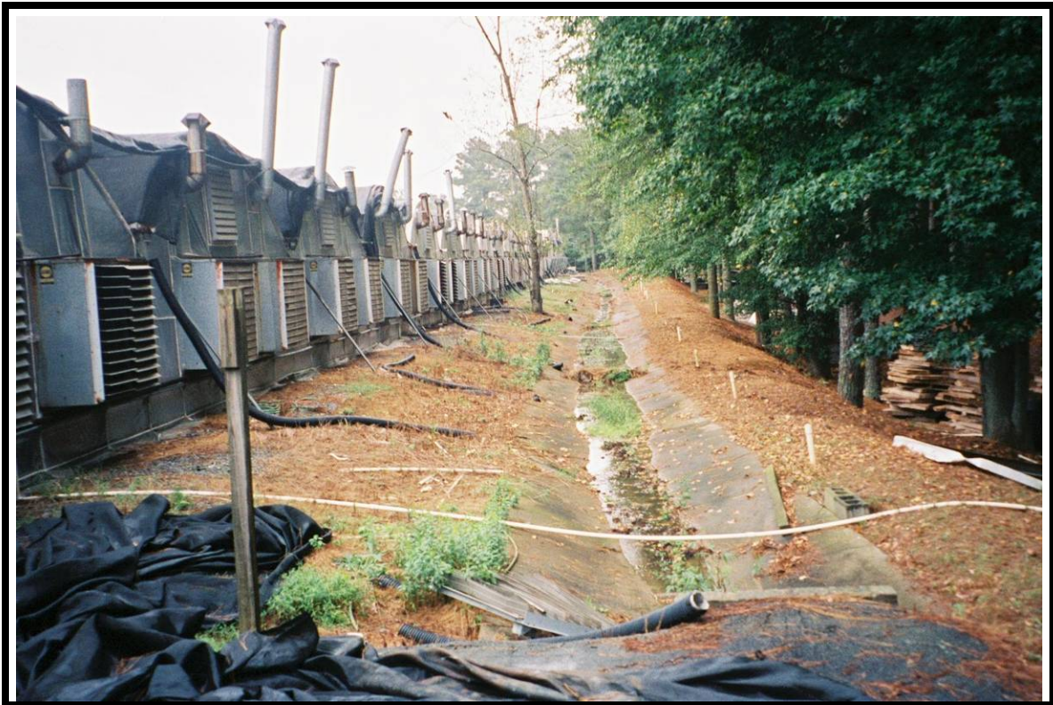
6. View of the concrete flumes for drainage located to the south of the sunscreen-covered areas.
