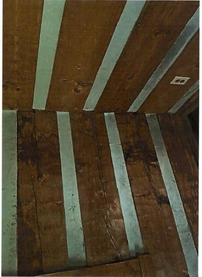
Water penetration in front office area
