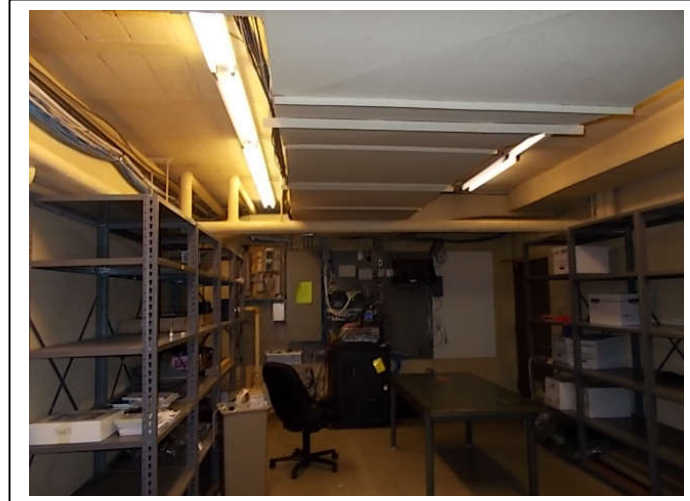
View Of: Lower level mechanical office, ACM fittings observed
