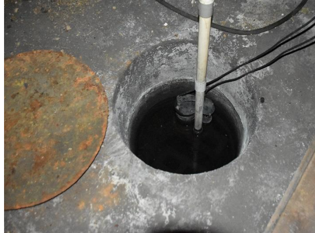
Representative Sump in Basement
