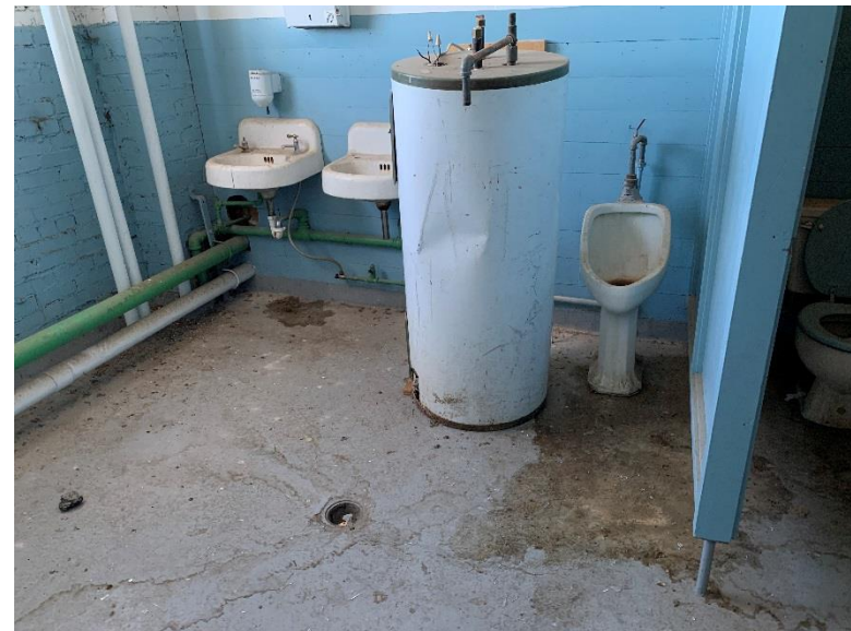
Restroom Area in Northern Portion of Warehouse, 2 nd Floor – View to South
