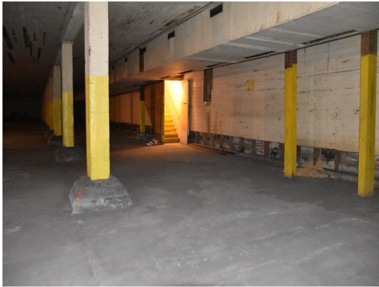
Representative Air Ducting System in Warehouse
