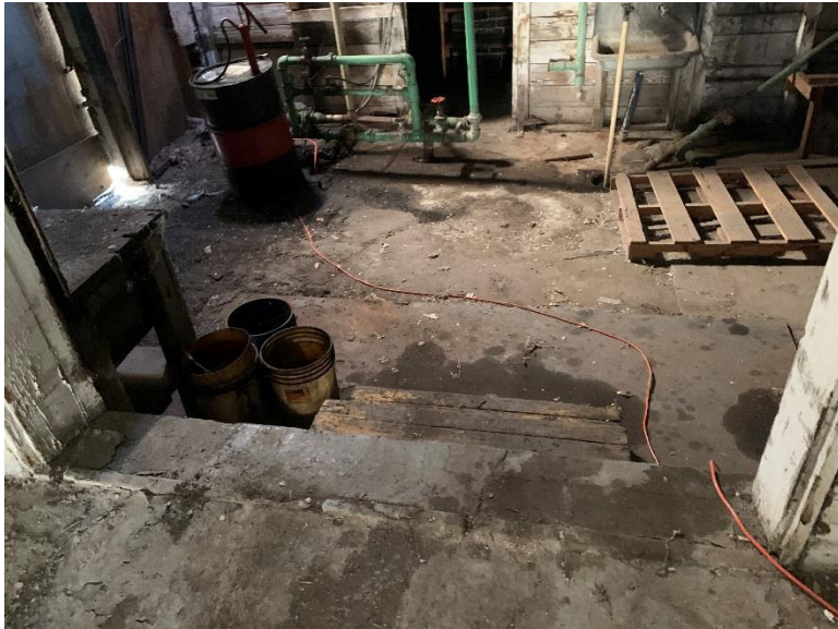
Eastern Portion of Mechanical Room, Well Visible and Remnant 55-Gallon Drum in Top Left, Floor Drain Present in Top Right – View to East
