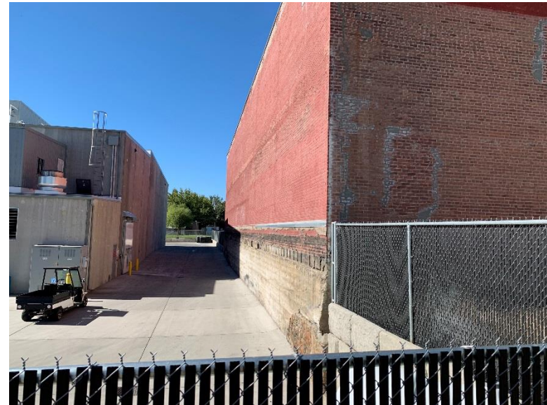
View along Subject Site Southern Property Boundary, Adjoining Property in the Left of Frame – View to West
