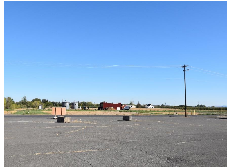
Subject Site Asphalt Lot and Adjoining Undeveloped Property in Background – View to East
