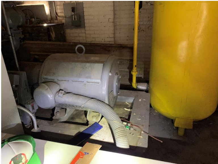
Representative Remnant Refrigeration System Pump
