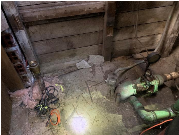
Well Located in Mechanical Building
