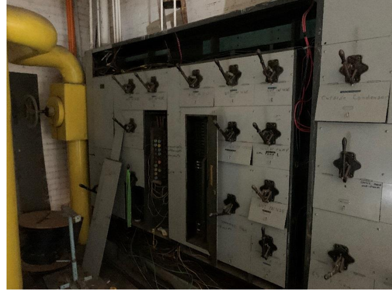
Electrical Panels along Western Interior Wall of Mechanical Building
