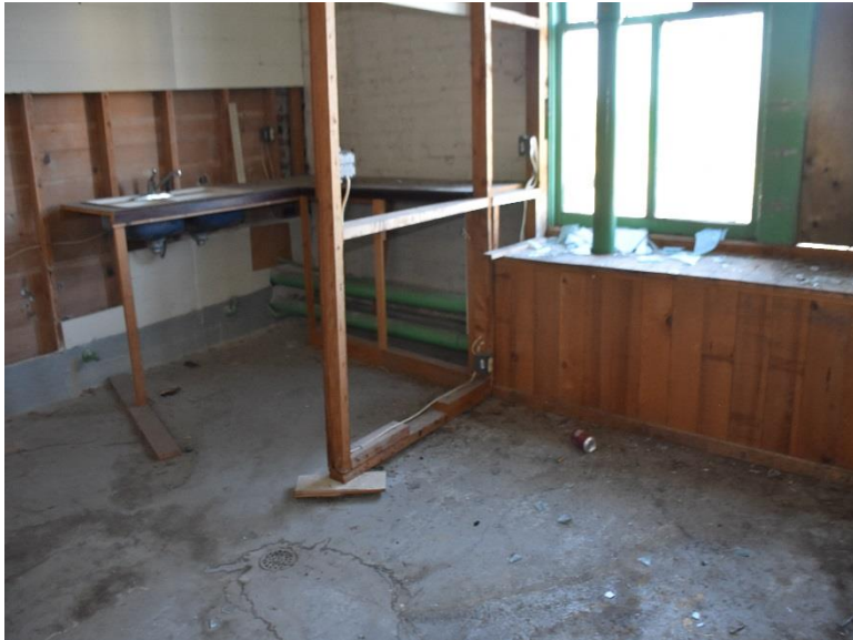
Restroom Area in Northern Portion of Warehouse, 2 nd Floor – View to East
