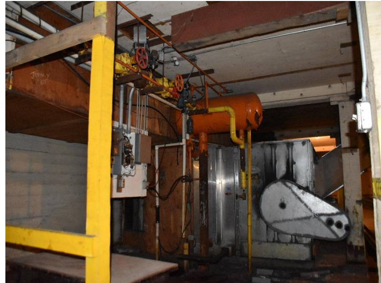
Representative Air Handling Unit in Basement
