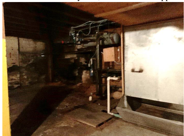
Representative Air Handling Unit and Equipment
