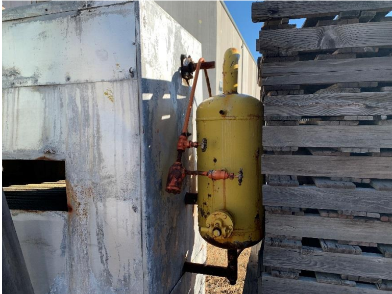
Remnant air handling unit in southwest portion of Subject Site – View to South
