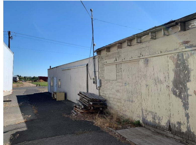
Mechanical Building North Exterior Wall, Division of Original Building (Western Portion) and Newer Construction (Eastern Portion) – View to Southeast
