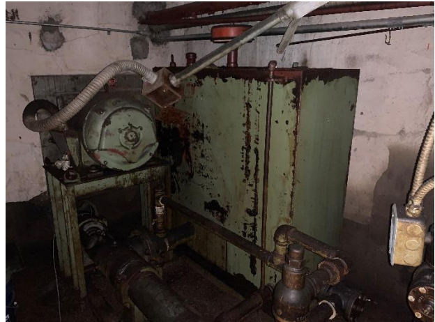
Elevator Hydraulic System
