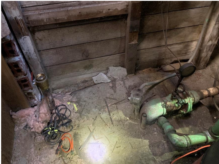
Well Located in Northeastern Portion of Mechanical Room – View to East
