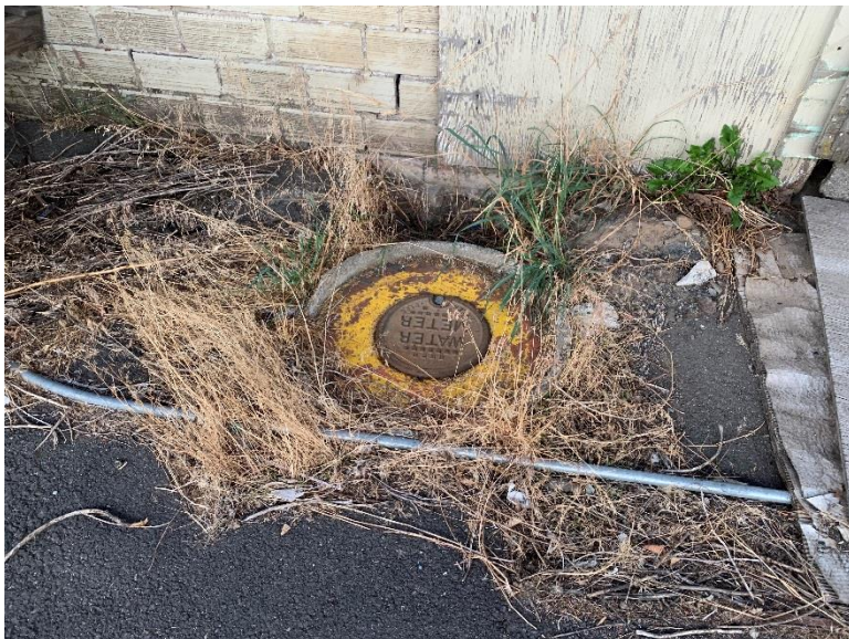
City Water Meter Present on North Side of Mechanical Building Immediately Opposite Well Location in Interior of Building
