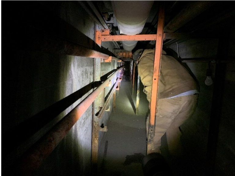
Interior of Refrigeration Line Tunnel Leading to Warehouse Building Basement – View to West
