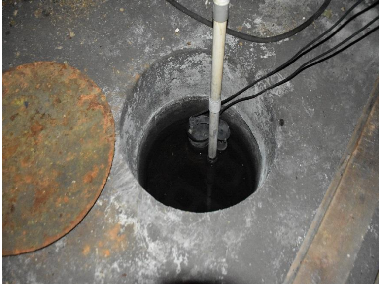
Representative Sump in Basement Adjacent to Air Handling Unit
