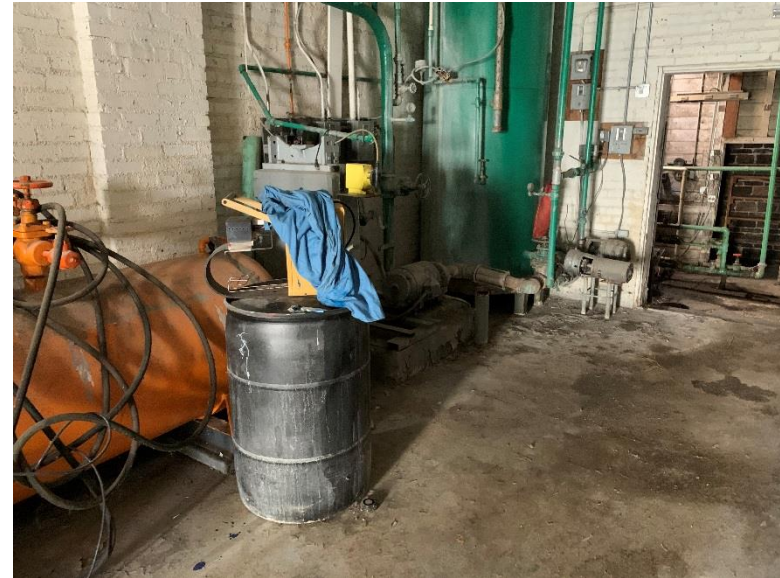
Representative Remnant Refrigeration System Tanks and Components
