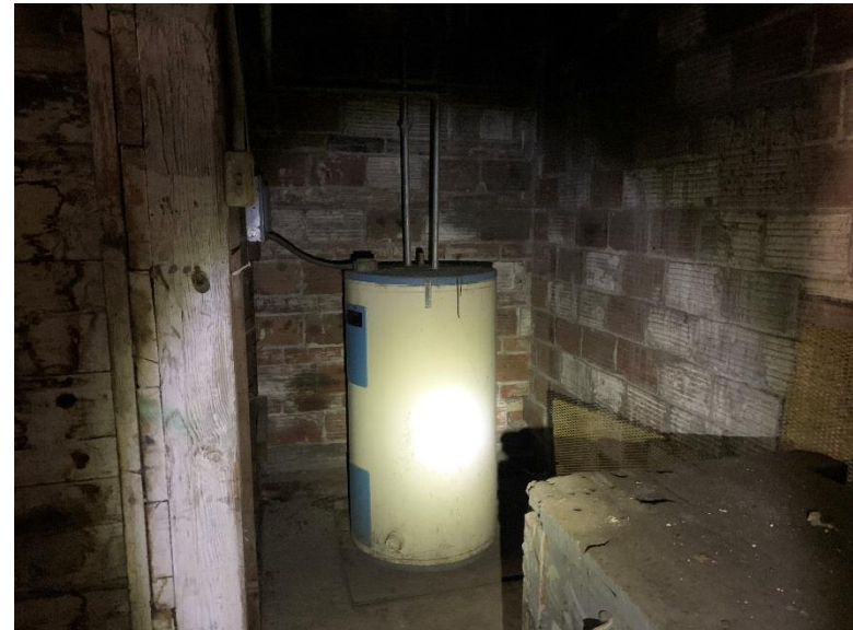
Hot Water Heater in Southeast Corner of Mechanical Room
