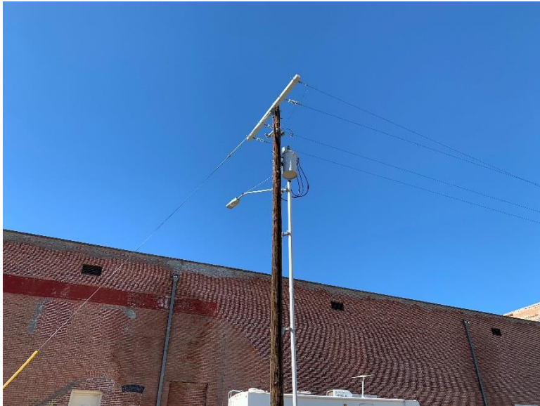
Pole Mounted Transformer Located near the Warehouse in the Southeastern Portion of the Subject Site
