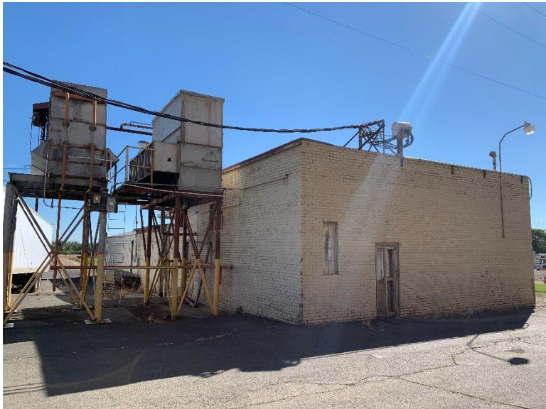
Mechanical Building in the Eastern Portion of Subject Site – View to Southeast
