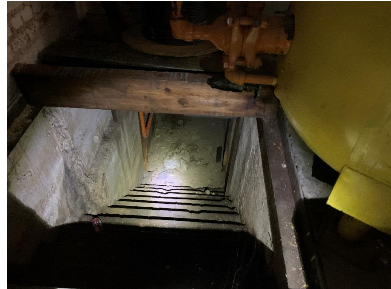
Access to Refrigeration Line Tunnel in Southwest Interior Corner of Mechanical Building, Leading to Warehouse Building Basement
