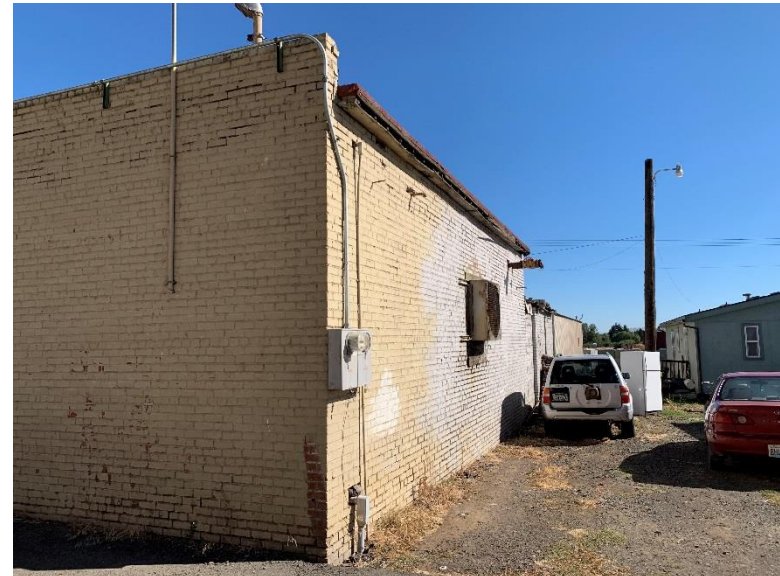
Mechanical Building in the Eastern Portion of Subject Site – View to Northeast
