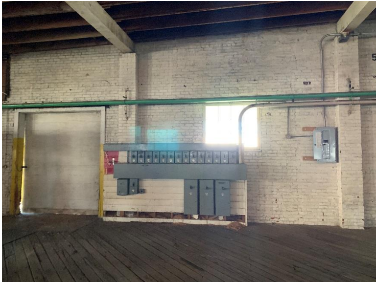
Electrical Panels in Northern Portion of Warehouse, Main Floor – View to East
