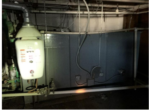
Water Treatment Tank on Main Floor
