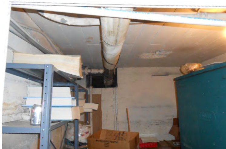
TSI in elevator room.
