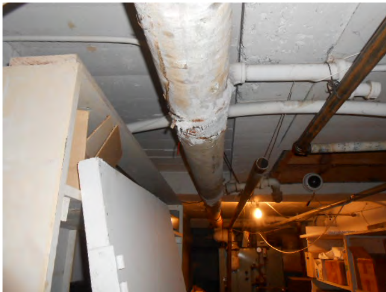
Same as above, stop at fiberglass TSI.
