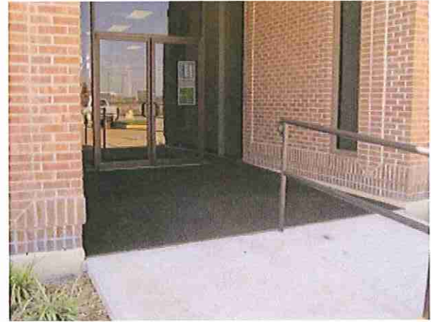
Photo #16 Exterior carpet mastic (yellow).
