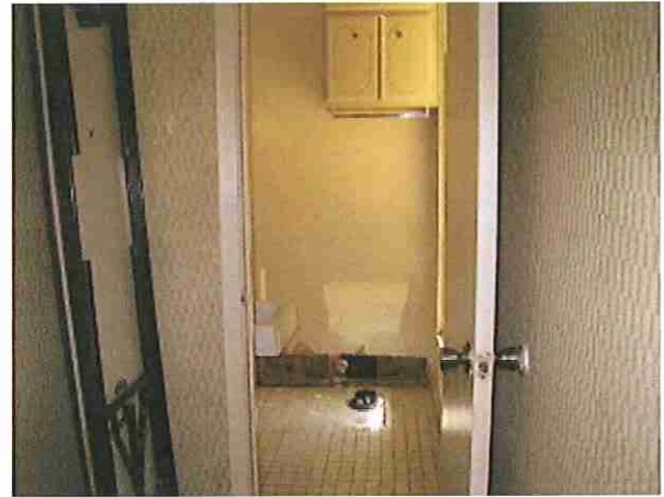
Photo #14 Grout (gray) associated with ceramic floor tile and wall texture/drywall/joint compound (beige, semi-smooth).
