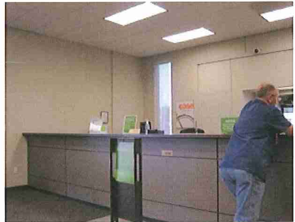
Photo #2 Lobby and teller line, light fixtures set in 2' x 2' Ceiling tile (white, pinholes, indents) system
