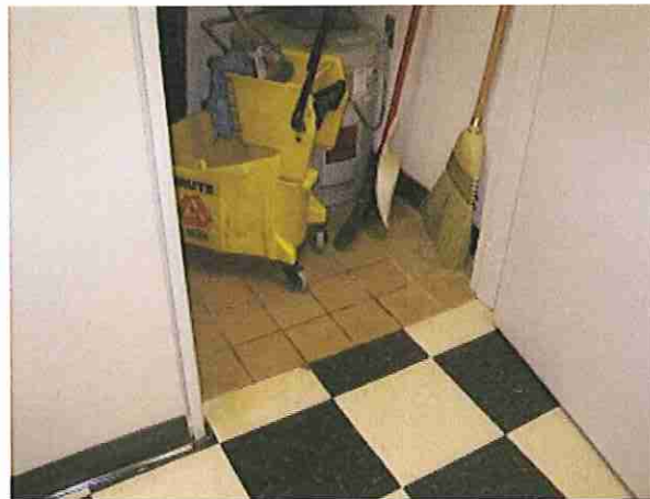
Photo #11 Grout (dark gray/black) associated with ceramic floor tile.
