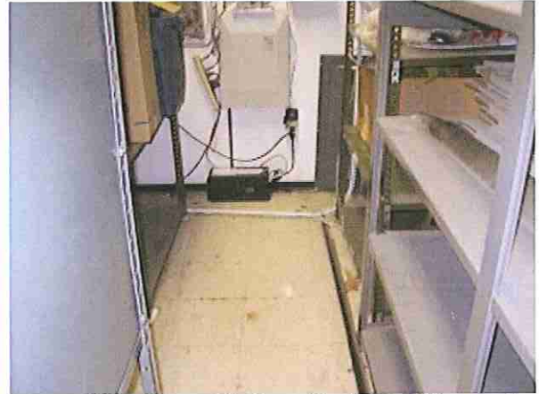
Photo #10 12" x 12" floor tile (tan) with mastic (black).
