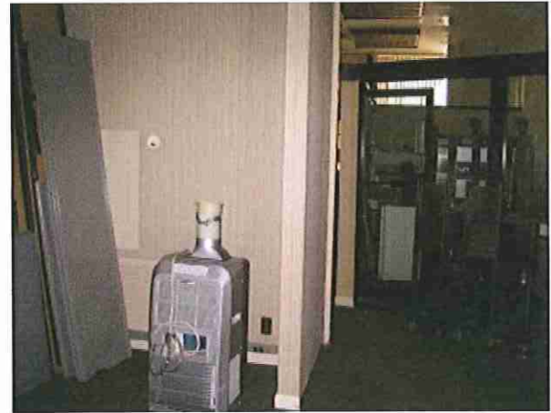
Photo #12 Drywall/joint compound associated with wall covering (multi-color)..
