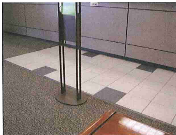
Photo #5 Grout (gray) associated with ceramic floor tile and carpet mastic (tan).
