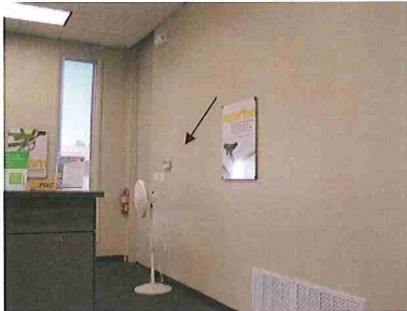
Photo #3 Thermostat on wall texture/drywall/joint compound (tan, semi-smooth)
