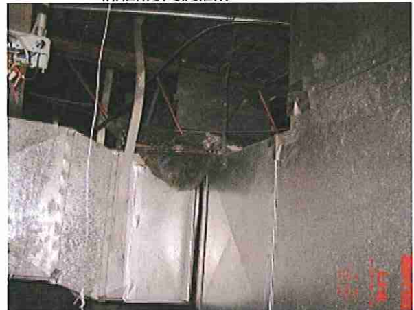
Photo #4 Duct work located above the lay-in ceiling tile system.
