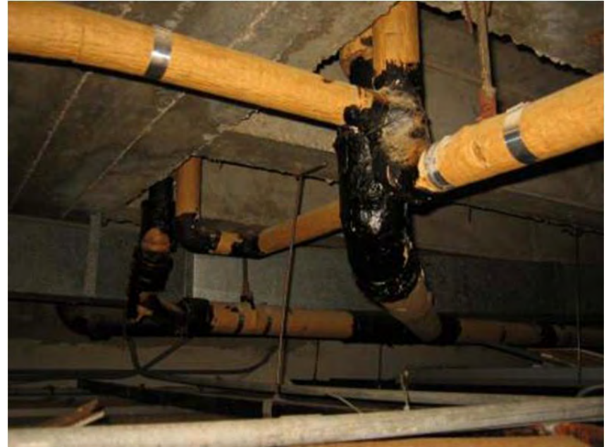
Photo 10: View above ceiling on 2 nd floor. Black pipe mastic was identified as ACM in August 2010.
