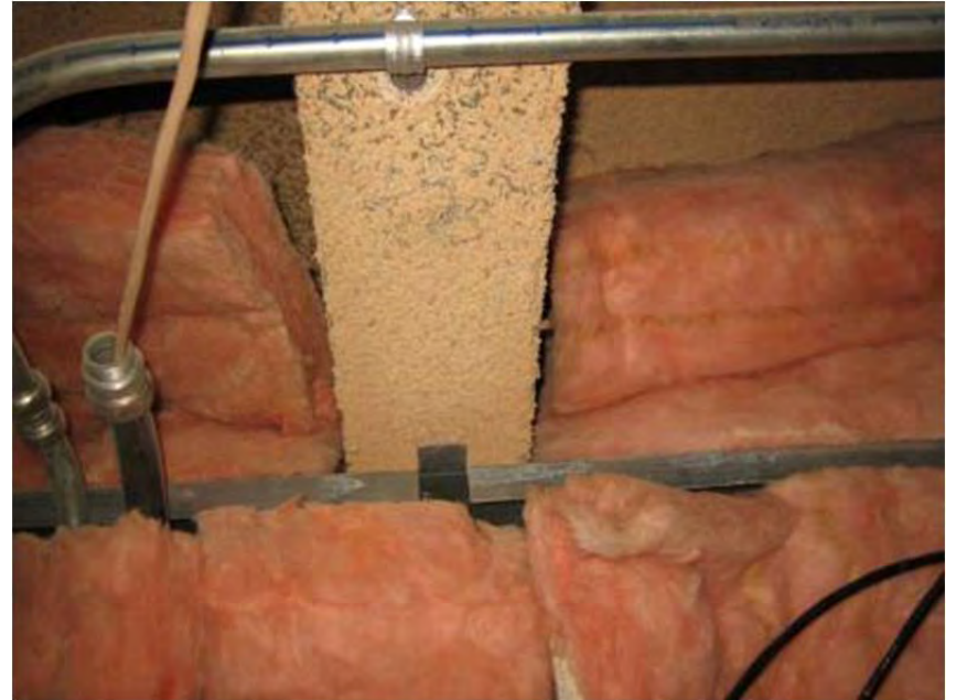
Photo 6: ACM fireproofing in 1 st floor front office area.
