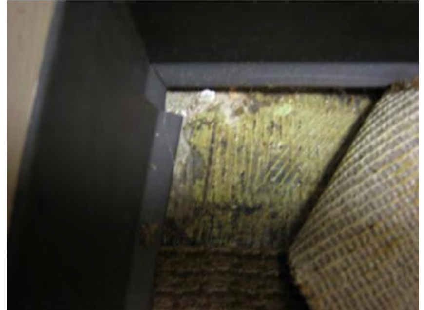
Photo 2: ACM black mastic beneath carpet, green mastic is non-ACM.
