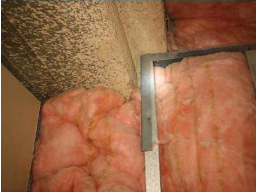
Photo 5: ACM fireproofing in 1 st floor front office area.
