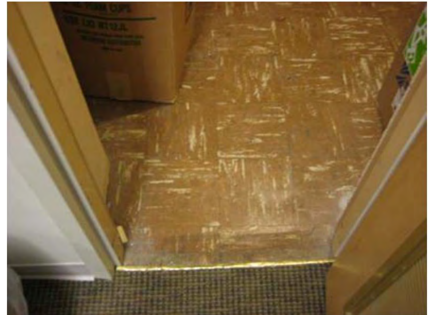
Photo 4: ACM 9"x9" floor tile brown with white streaks.
