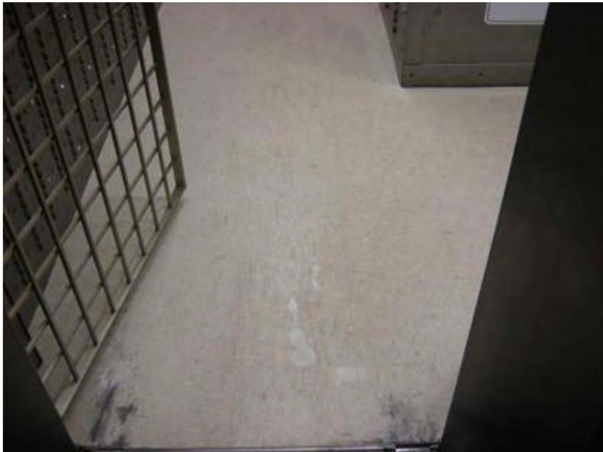
Photo 3: Non-ACM 12"x12" floor tile in 2 nd floor vault, 2 nd layer flooring is ACM.
