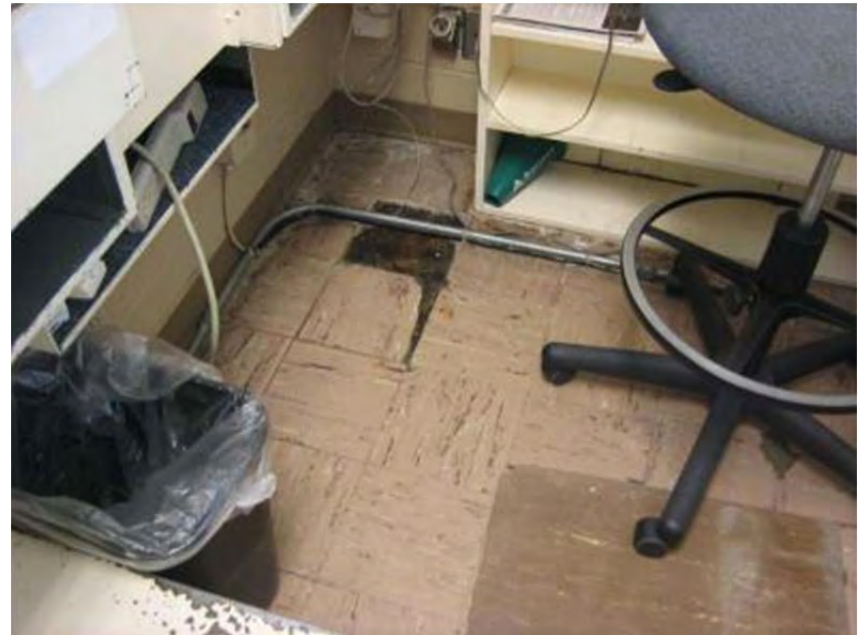
Photo 8: ACM 9"x9" floor tile in drive-through teller booths.
