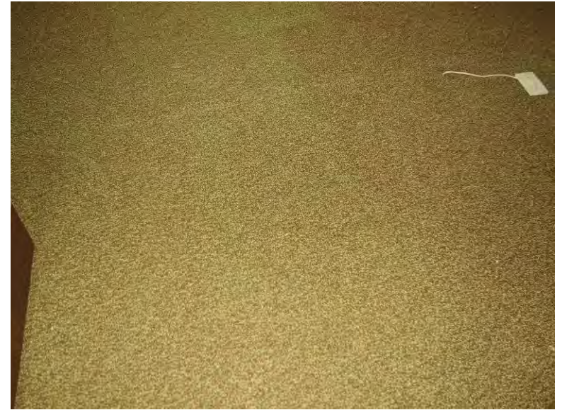
Photo 2: An example view of carpet that was glued to the floor with mastic.
