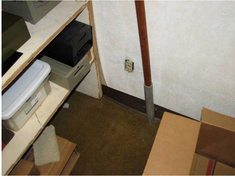
Photo 5: An example view of plaster and vinyl cove base in the structure.
