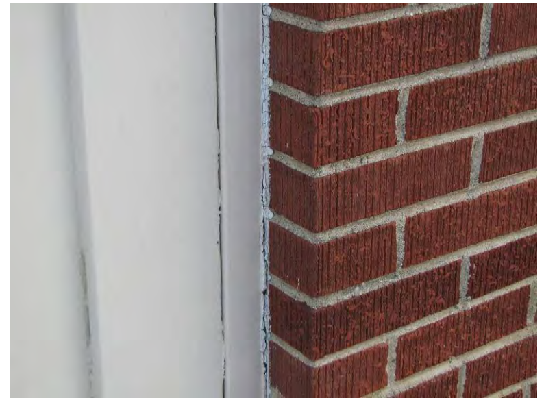
Photo 8: An example view of asbestos-containing white caulk on other sides of the building.
