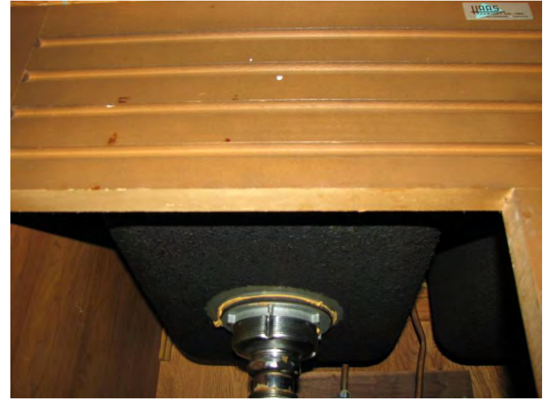
Photo 6: View of asbestos-containing black sink undercoating in the kitchenette.
