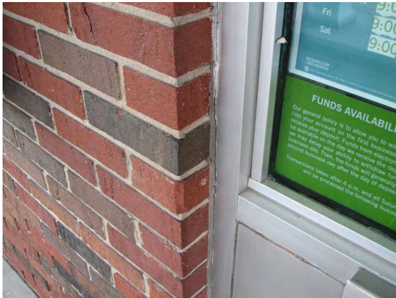
Photo 7: View of asbestos-containing gray caulk on the north side of the building.
