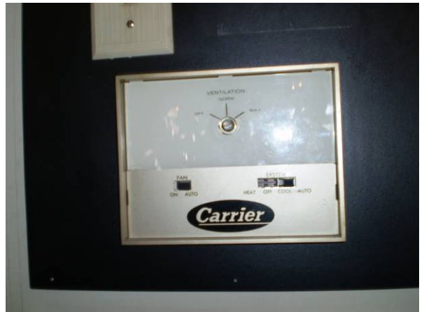
Photo #30 Thermostat on Wood in Lobby
