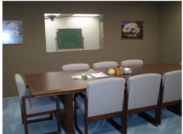
Photo #46 Conference Room Showing ACM Gypsum Wallboard Joint Compound (HA#20)
