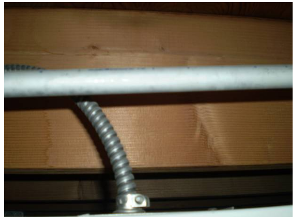
Photo #28 Above DCT in Office 3
