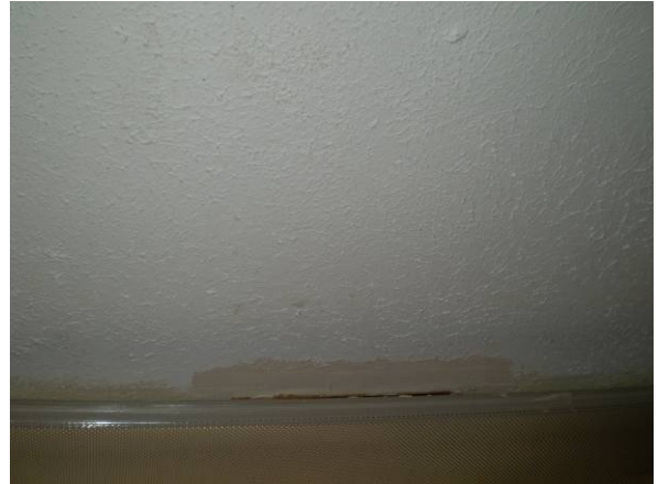
Photo #10 ACM Textured Ceiling (HA#16)
