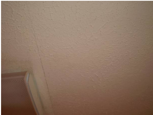
Photo #23 ACM Textured Ceiling, (HA#16)
