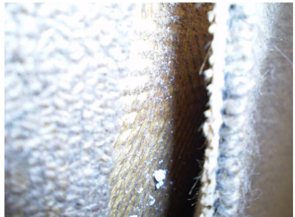
Photo #12 ACM Wall Carpet Mastic, Brown (HA#6)
