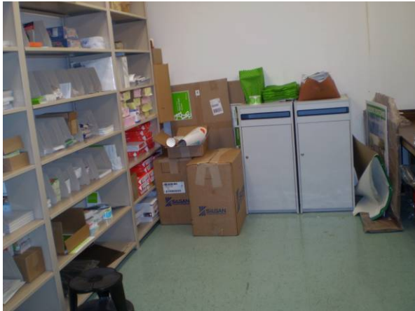
Photo #43 Office Storage with ACM Beige & Cream Vinyl Floor Tile (HA#2) under 12"x12" Mint Green Vinyl Floor Tile (HA#1)
