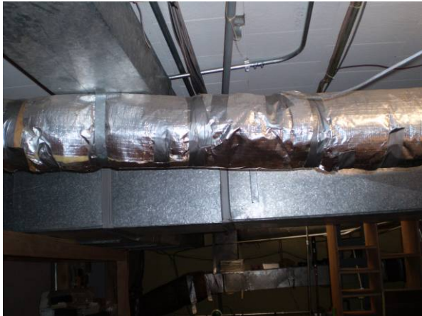
Photo #31 HVAC System in Attic
