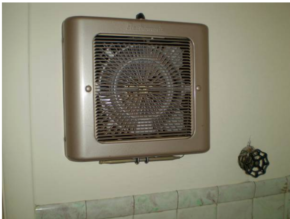
Photo #41 Fan on Wall of Bathroom
