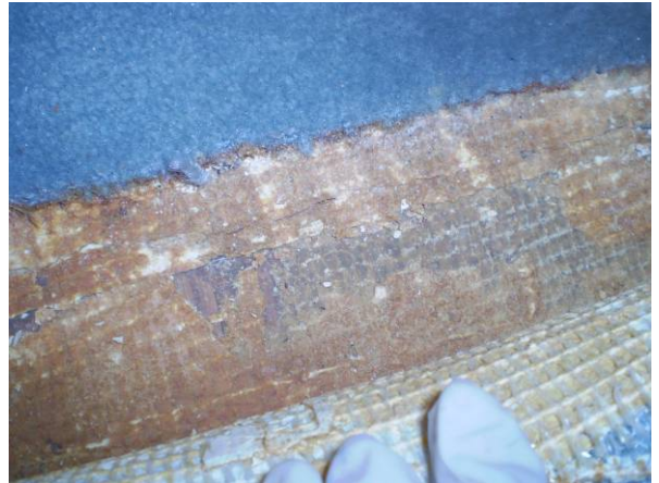
Photo #26 Beneath Carpet in Conference Room
