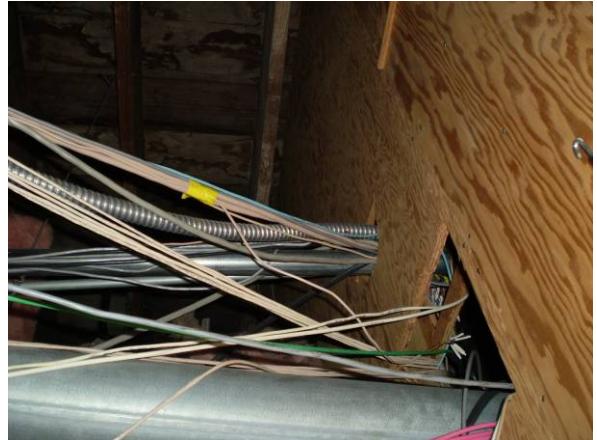
Photo #20 Above Dropped Ceiling Tile in Teller Area
