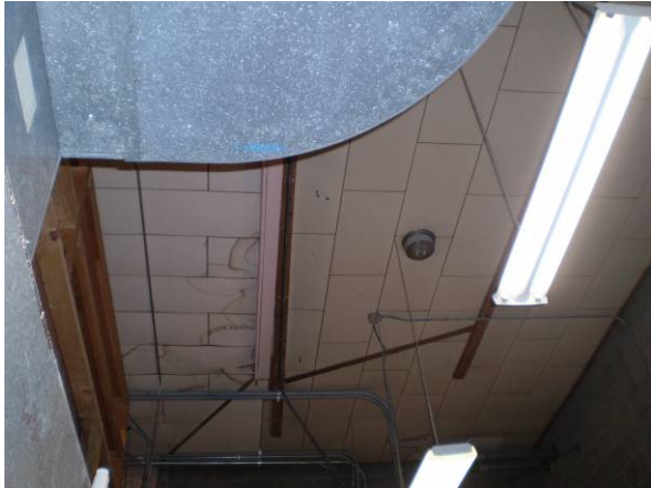
Photo #9 4'x2' Ceiling Panels with Water Damage in Attic (HA#8)
