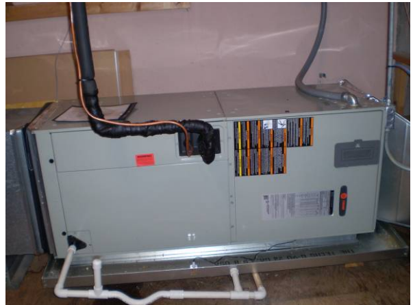
Photo #40 HVAC Unit in Attic
