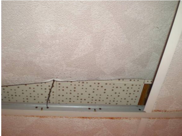
Photo #21 Above Fiberglass Ceiling Tile in Office 6 Showing HA#7
