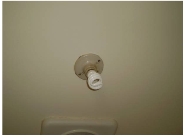
Photo #38 Bathroom Lighting
