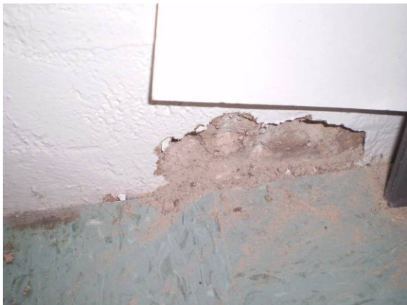
Photo #17 Plaster Skim Coat (HA#21)
