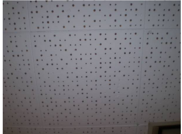
Photo #8 12"x12" Ceiling Tile with Large Holes (HA#7)
