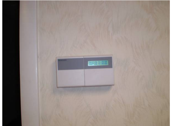
Photo #22 Thermostat on Gypsum Wallboard with Wallpaper in Conference Room
