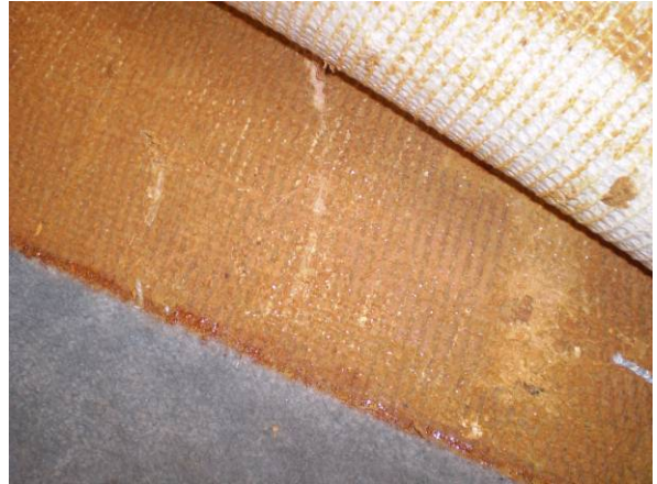
Photo #14 ACM Carpet Mastic, Brown (HA#18)
