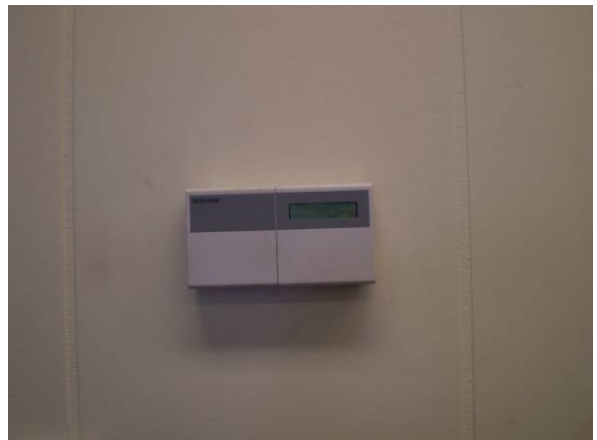
Photo #18 Thermostat on Painted Wood Paneling in Teller Area
