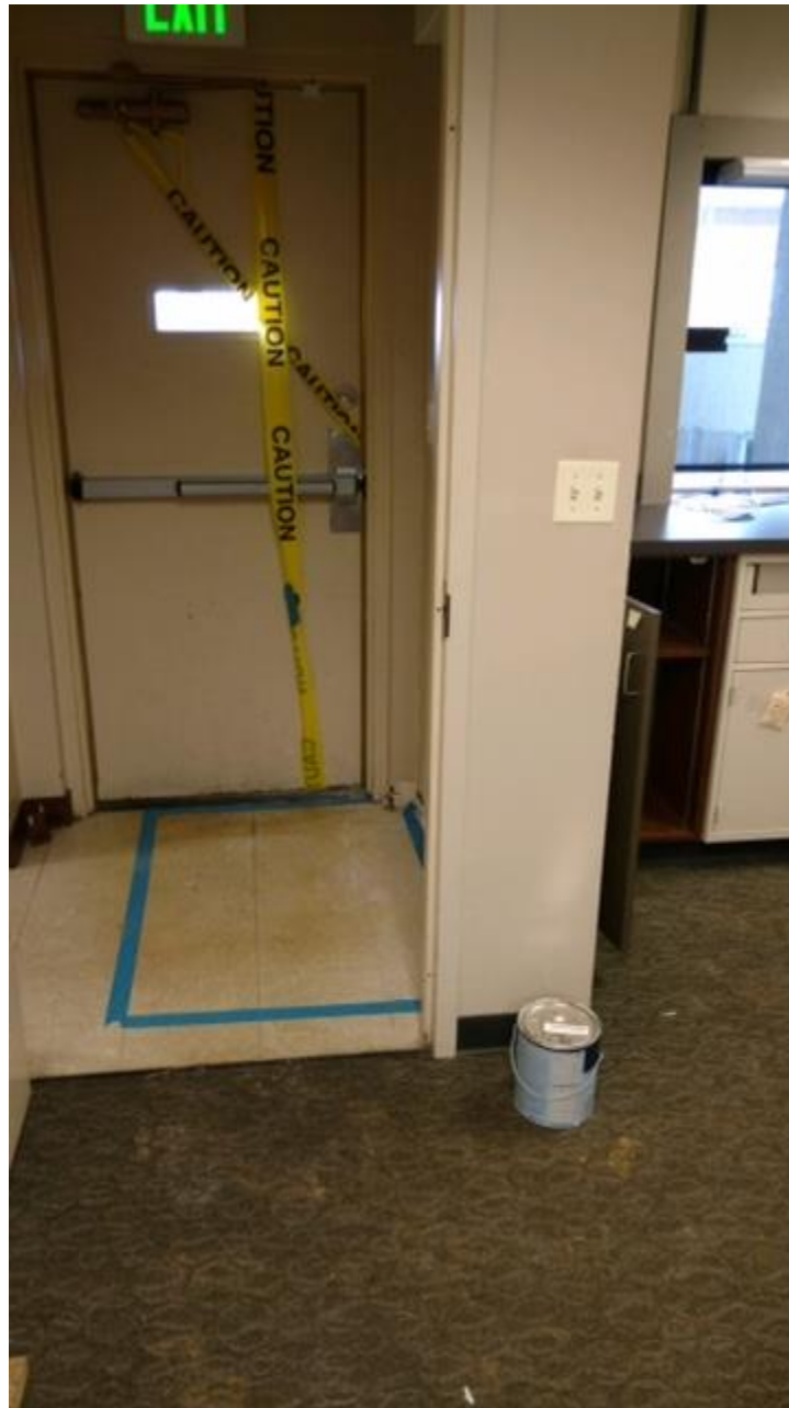
Photo 1: View of vinyl floor tile with ACM mastic indicating extent of removal.
