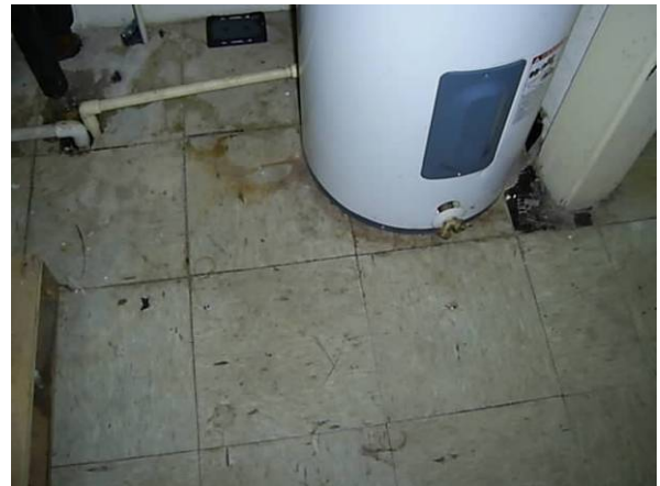
Photo #2 12x12 gray floor tile mastic – black located in the mechanical room and rear stairwell.
