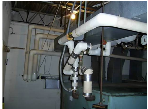
Photo #4 Yellow fiberglass pipe insulation white backing in mechanical room.
