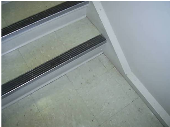
Photo #3 12x12 gray floor tile mastic – black located in the mechanical room and rear stairwell.
